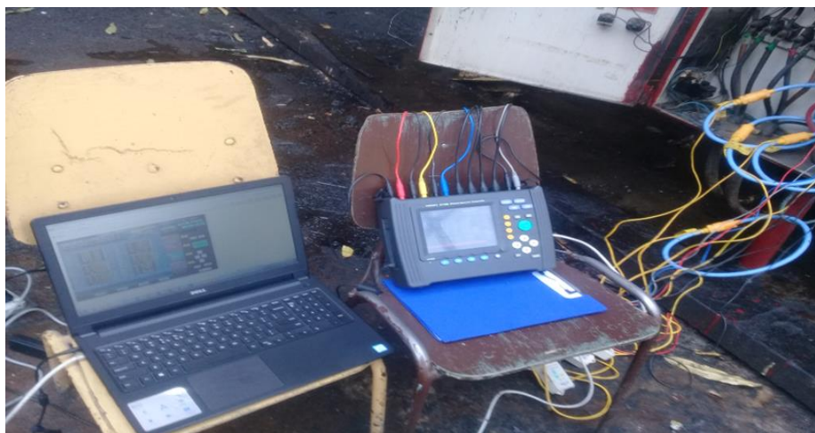
Figure 3.5: Measurement connection on 90 KW rating induction motor.
