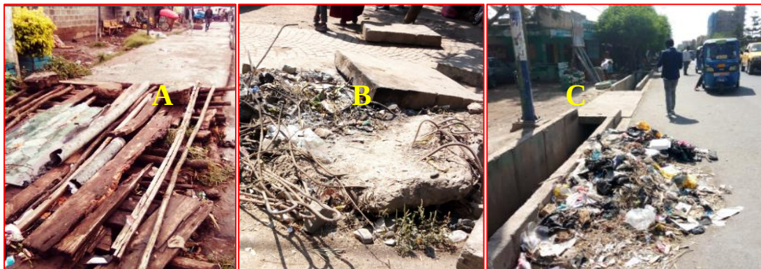
Figure 4.6. Problems in Infrastructure lines (Field survey, 2020).
