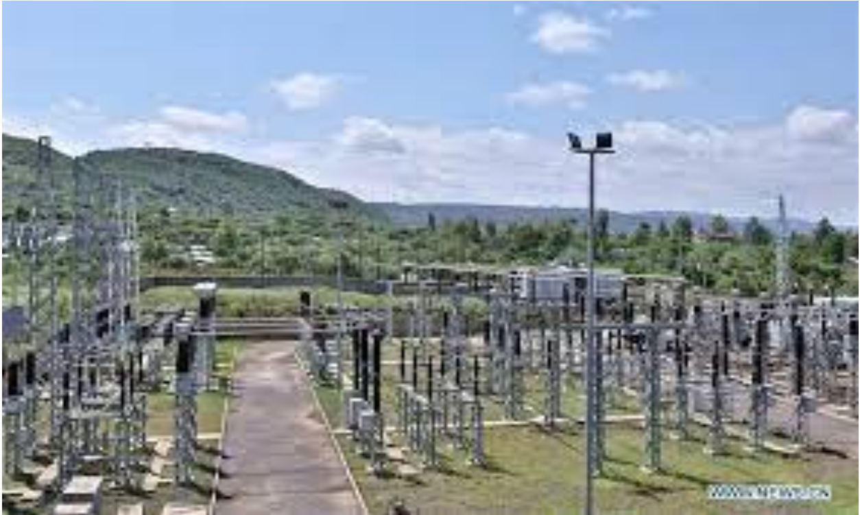
Fig 4.1 a, overview of Adama distribution Substation [GOOGLE IMAGE]
