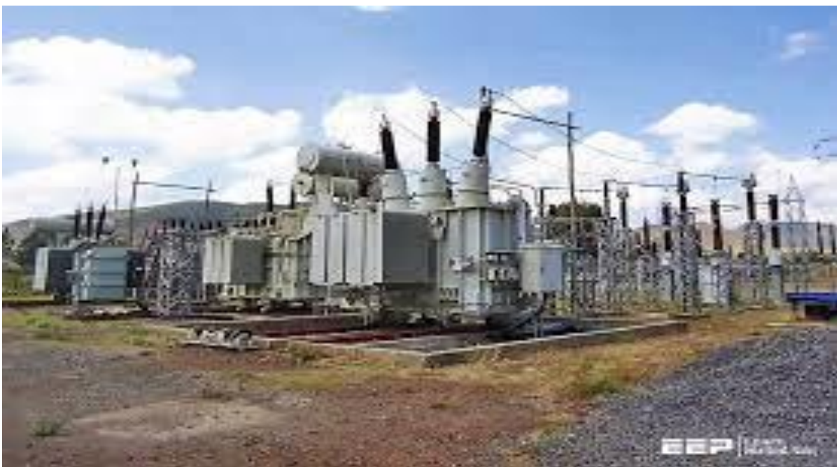
Fig 4.1 b overview of Adama distribution Substation [GOOGLE IMAGE]
