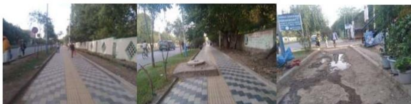
Figure 4-4: Bole segment sidewalk condition
