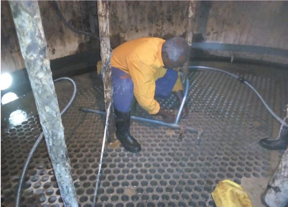
Appendix Figure 1 New WSSF heating calandria tubes manual cleaning system
