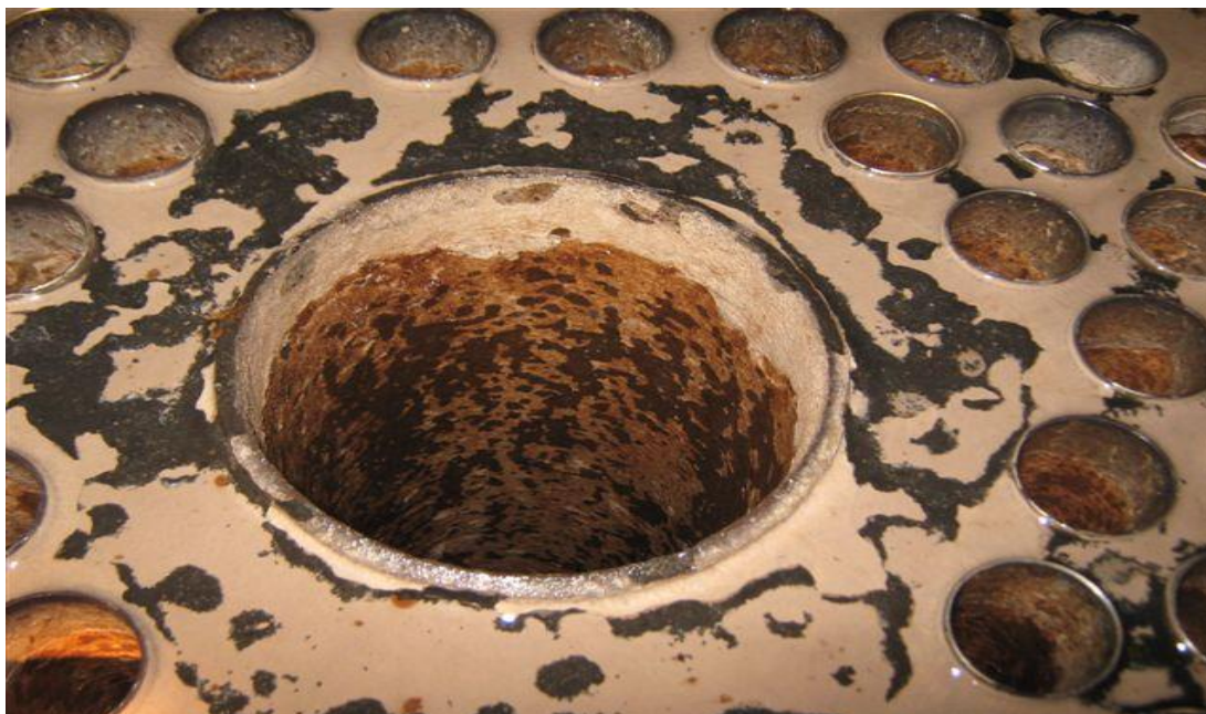
Figure 2.4 The inside of evaporator covered with scale (East, 2013)
