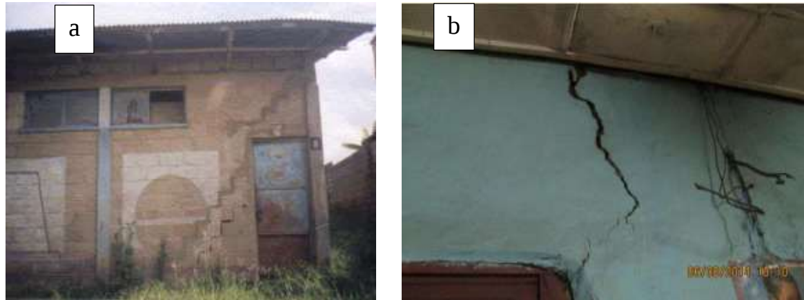
Figure 2.2: Typical damages due to soil swelling and shrinking characteristics show distress on lightweight structures (Tibebu, 2015)
