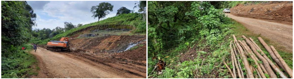
Figure 4.6: Landslide movement at station 69+180 – km 69+220 LHS
