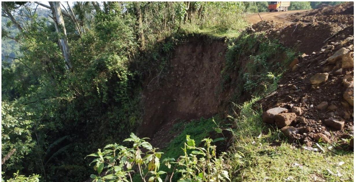
Figure 4.7: Landslide movement station from km 78+940-78+960 RHS
