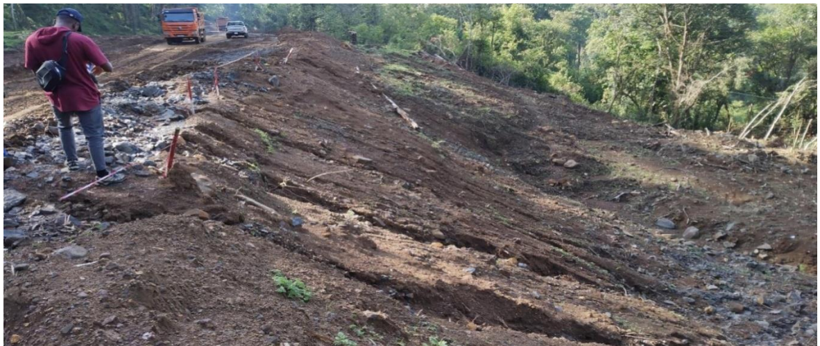
Figure 4.8: Landslide with settlement or movement station from 79+980 – km 80+010
