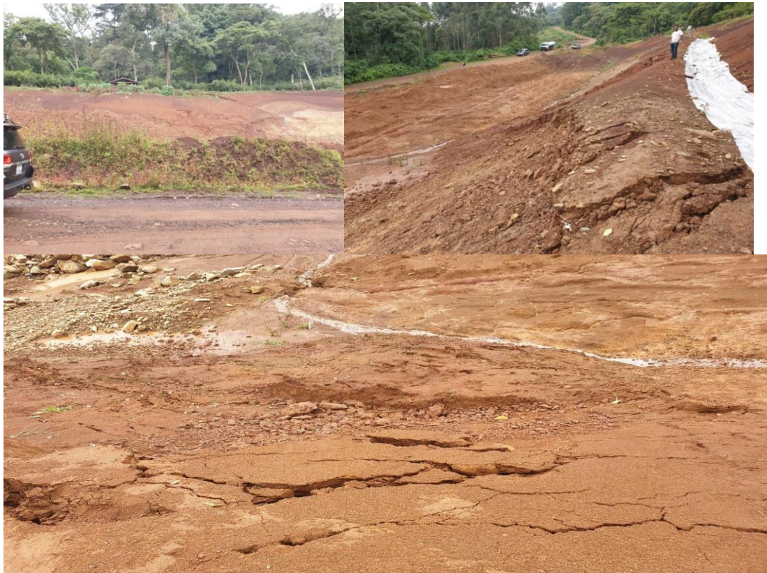
Figure 4.3: Landslide movement at station 45+350-45+440
