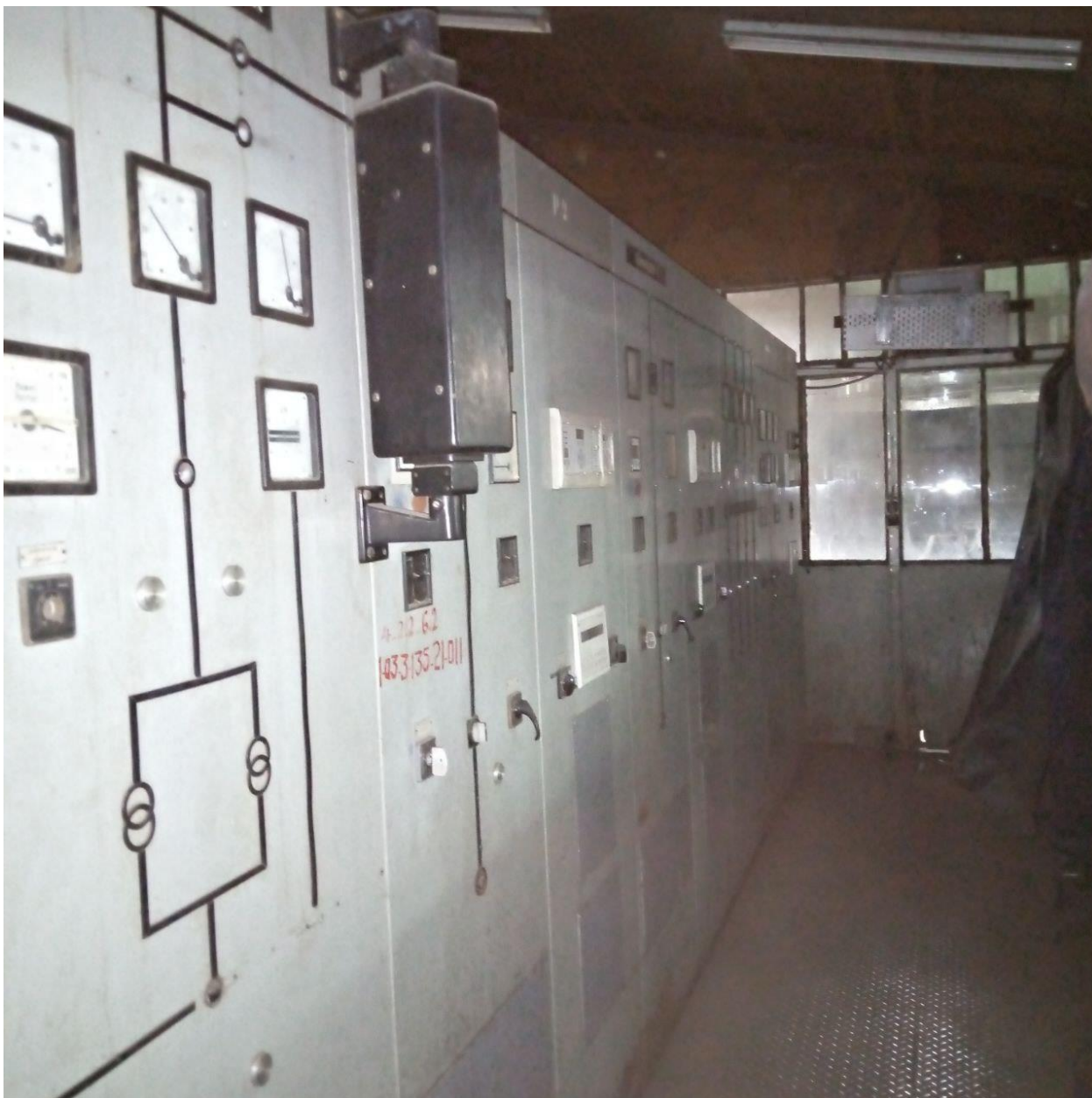
Figure 3.4:Metahara Sugar Factory partial view of power generation control room
