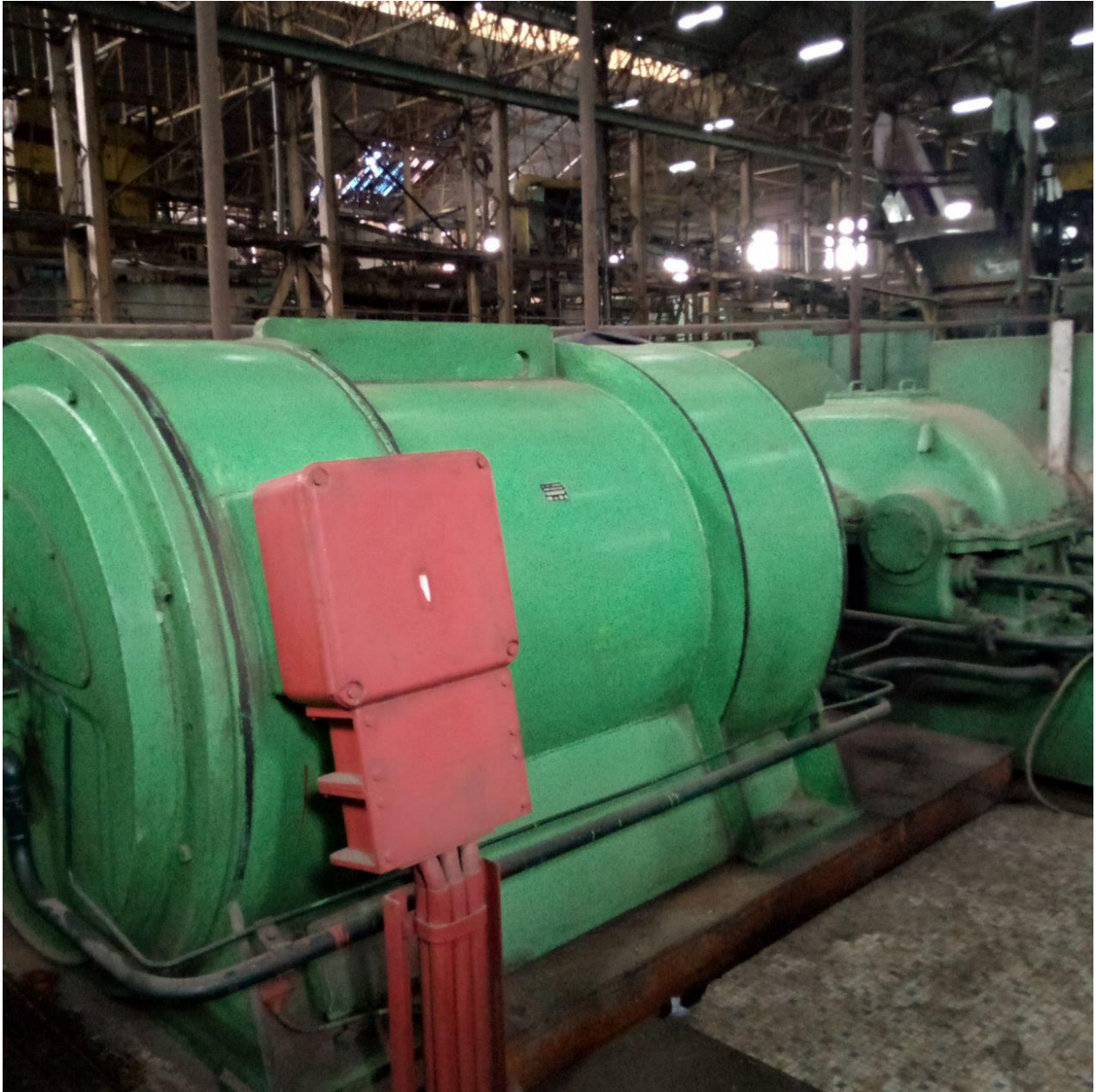
Figure 3.3:Metahara Sugar Factory side view of Alternator-gearbox-turbine assembly(unit #1)
