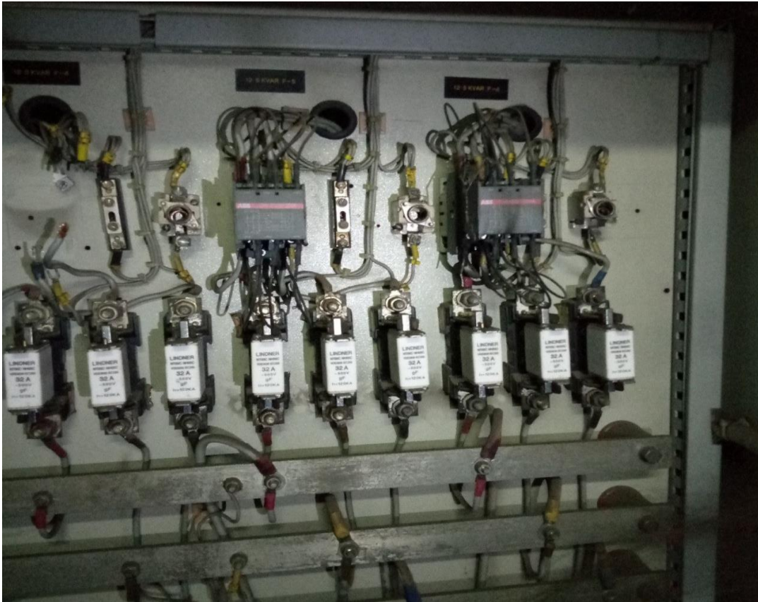
Figure 2.4: Burnt capacitor bank main fuses at Normivak panel in 2017 factory operation year
