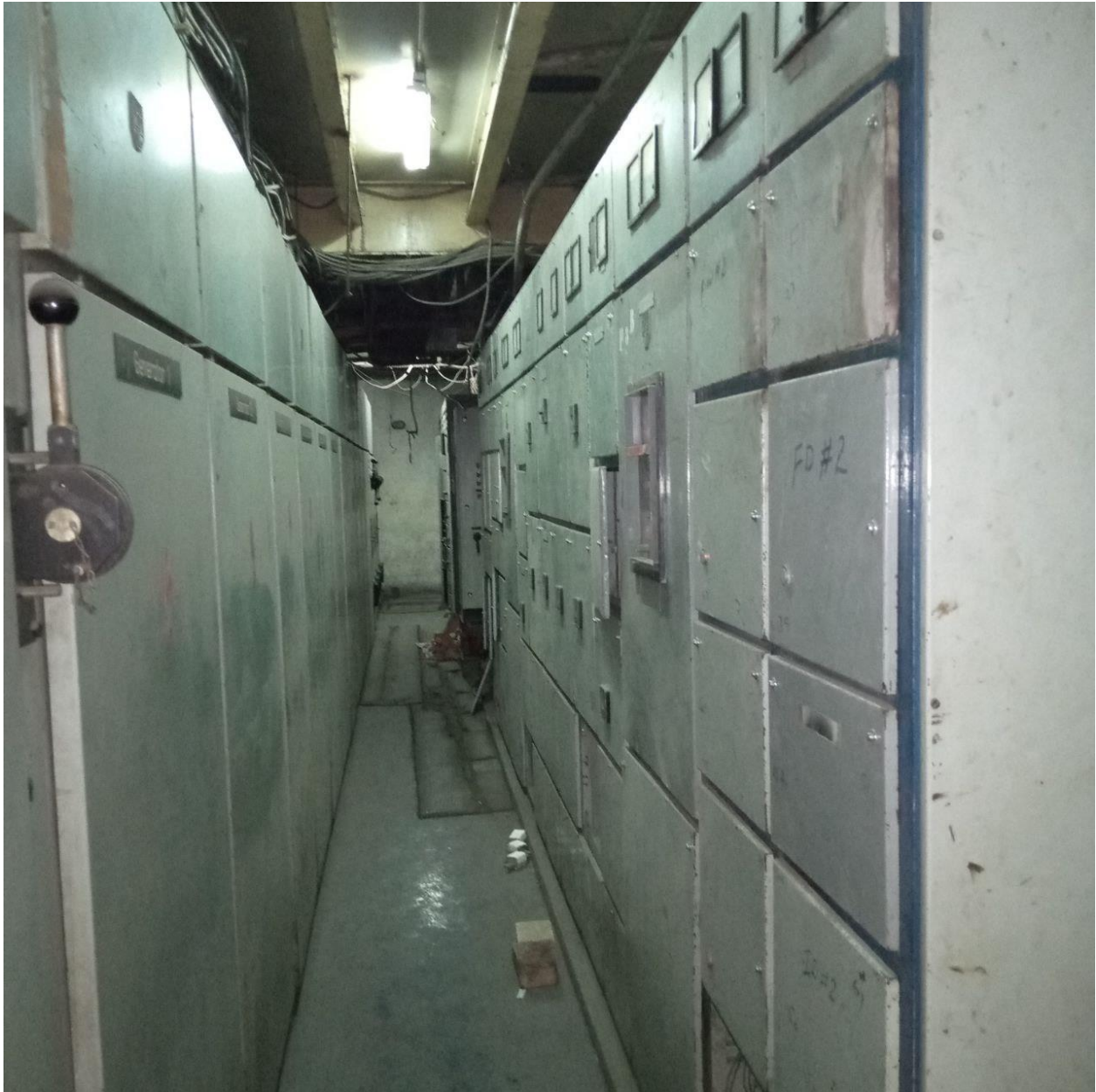
Figure 3.5: Metahara Sugar Factory partial view of power house
