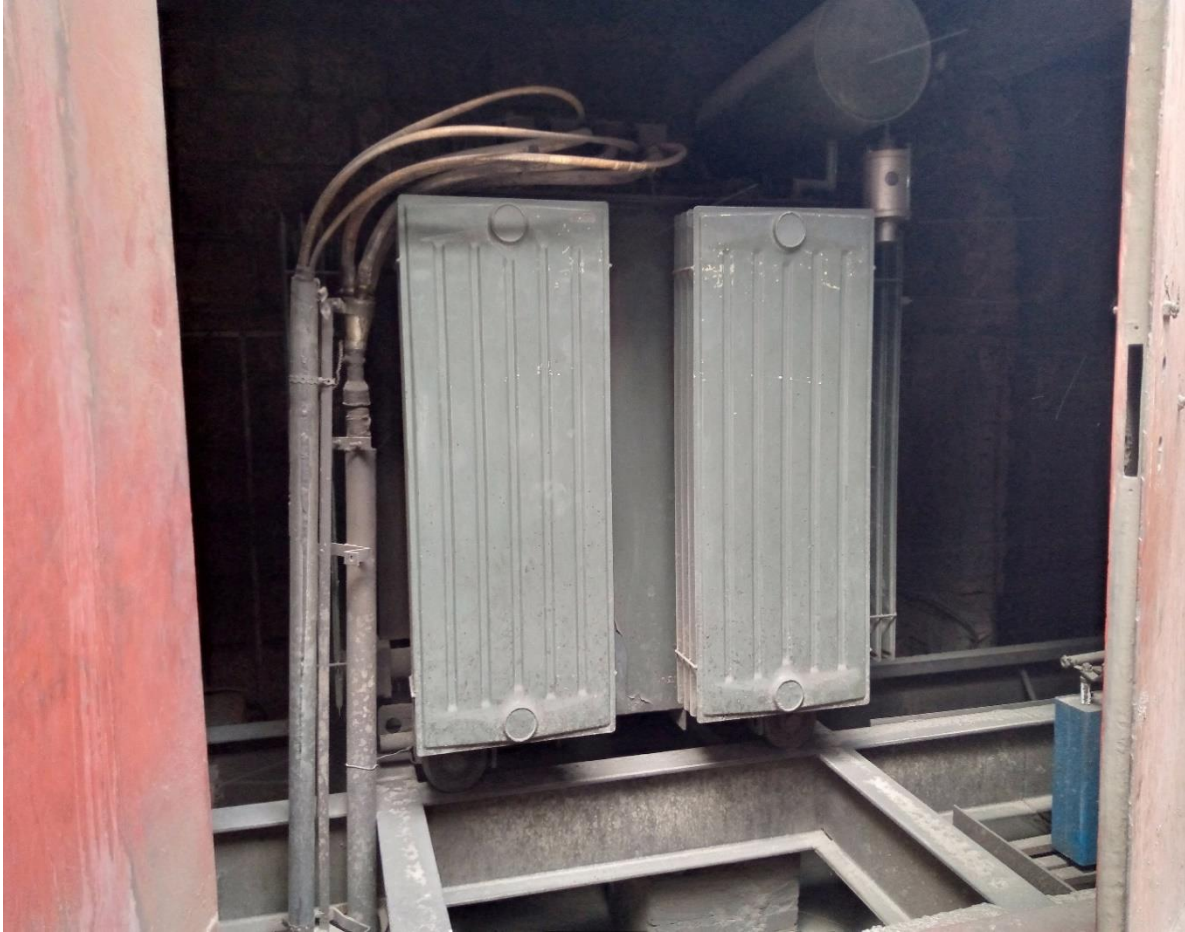
Figure 3.7: Indoor type distribution transformer#02 at boiler plant (Metahara Sugar Factory)
