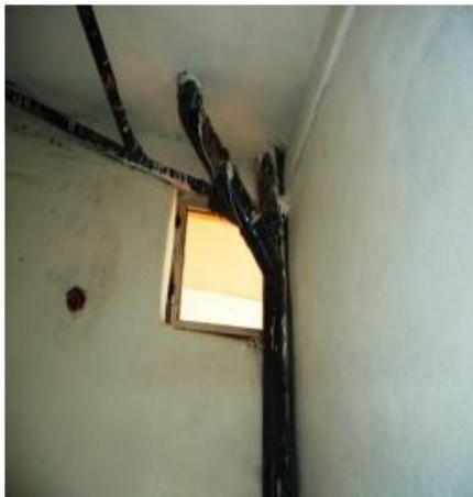
Figure 32 Poor plumbing (field work,2020)
