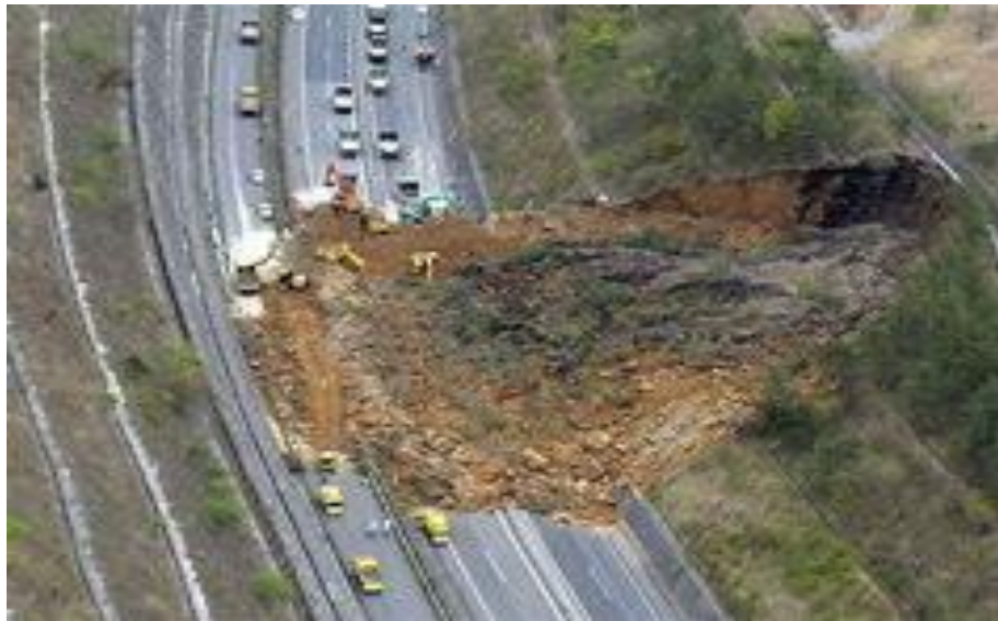
Fig 2.1 Source: USGS landslide hazard report (Oita Expressway, which was buried by a massive landslide in Japan seven years ago).
