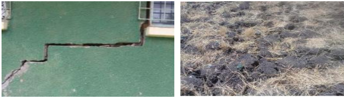
Figure 2. 5 Typical crack on expansive soil during the dry season (a) Diagonal cracks that develop below windows (b) ( Kassahun, 2006 )
