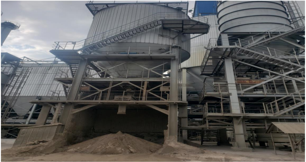
Figure 3. 6 photograph taken from power plant
