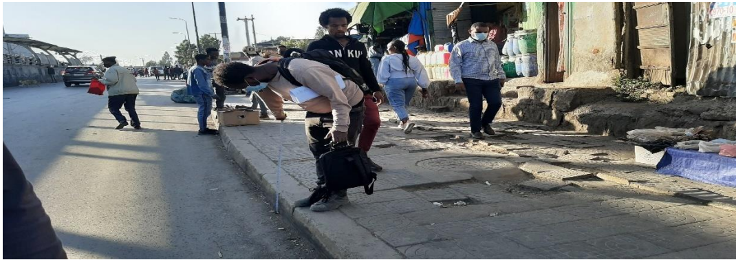
Figure 4. 24: Curb cuts with raised at zebra obstructing wheelchairs.
