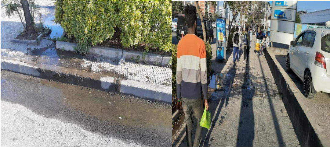
Figure 4. 34: Absence of proper drainage system and trees on walkways
