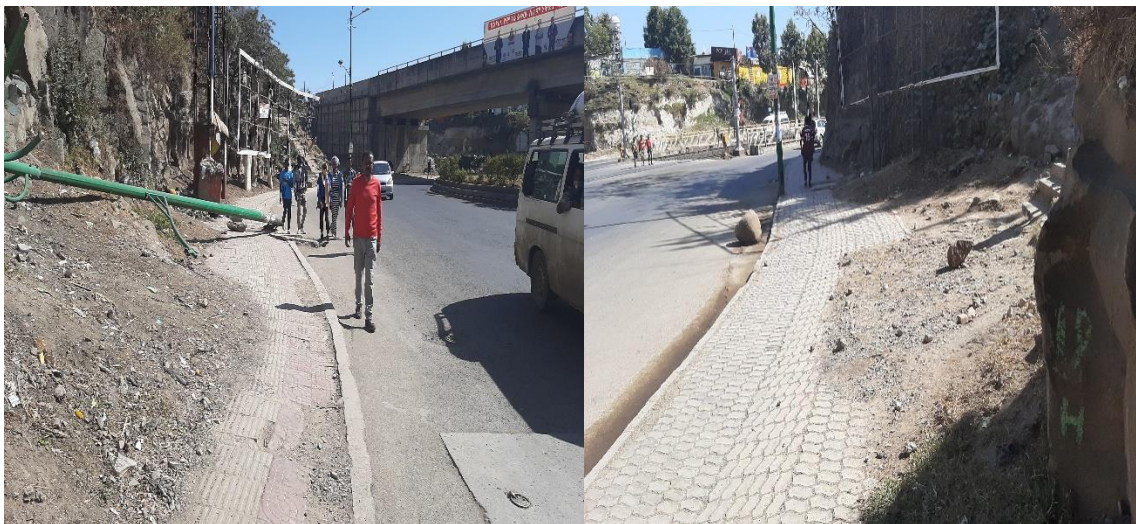
Figure 4. 17: Accumulation of waste materials that cover walkway and lack of tactile surface for visual disabled
