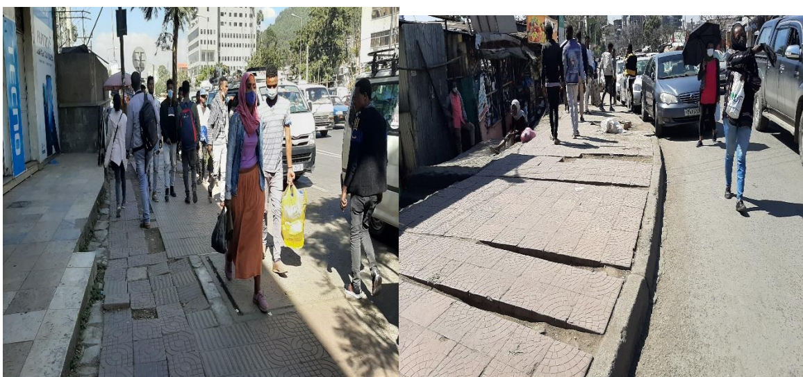
Figure 4. 68:Pop out tile from walkway and lack of tactile surface for visual disabled
