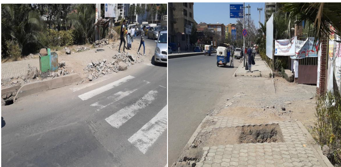
Figure 4. 11: Accumulation Waste materials and Open ditch Holes on Walkways
