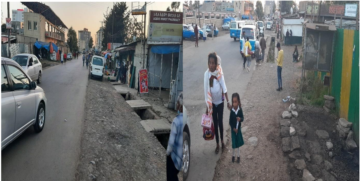
Figure 4. 27: Cracked road and lack of walkway access
