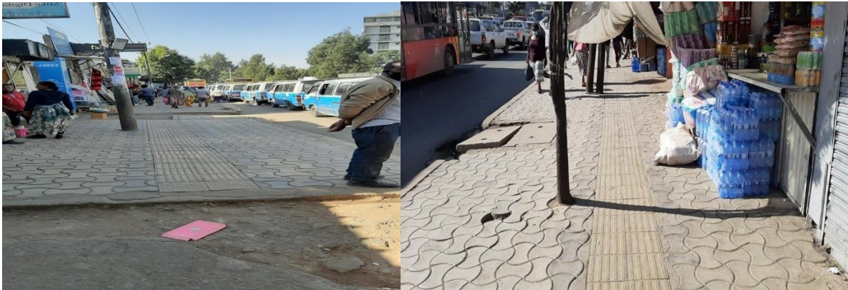
Figure 4. 28: Cracks of walkways and obstacle object on walkways
