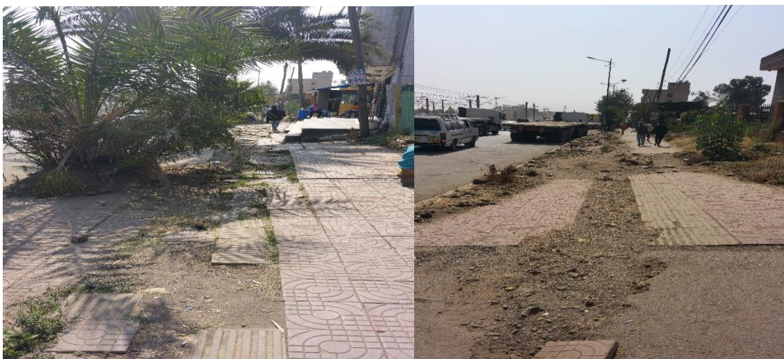
Figure 4. 49:Pop out and broken tile from walkways
