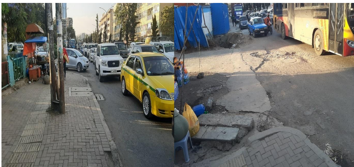
Figure 4. 19: Telephone pole and uncovered Hole on walkways
