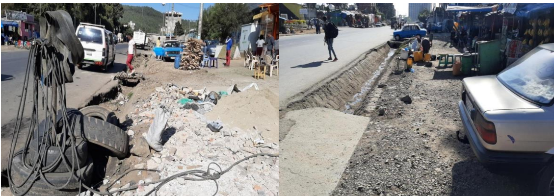
Figure 4. 29: accumulation of waste material on walkways and open ditch
