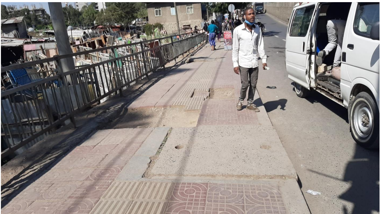
Figure 4. 83: Wrecked sidewalks and footpaths causing mobility difficulty for PwDs
