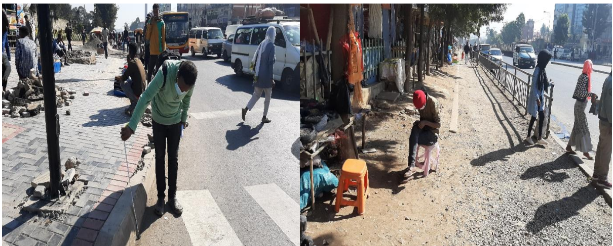
Figure 4. 48:Raised edge at zebra and improper walkways for disabled
