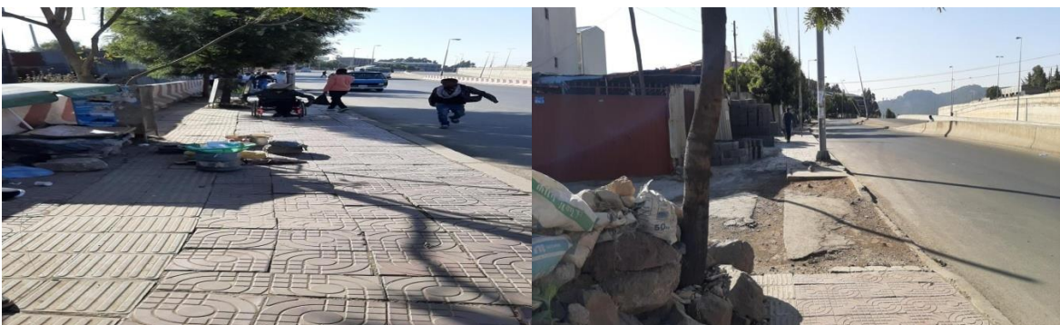
Figure 4. 30: Obstacle on tactile surface, improper walkways and uneven surface for wheelchair
