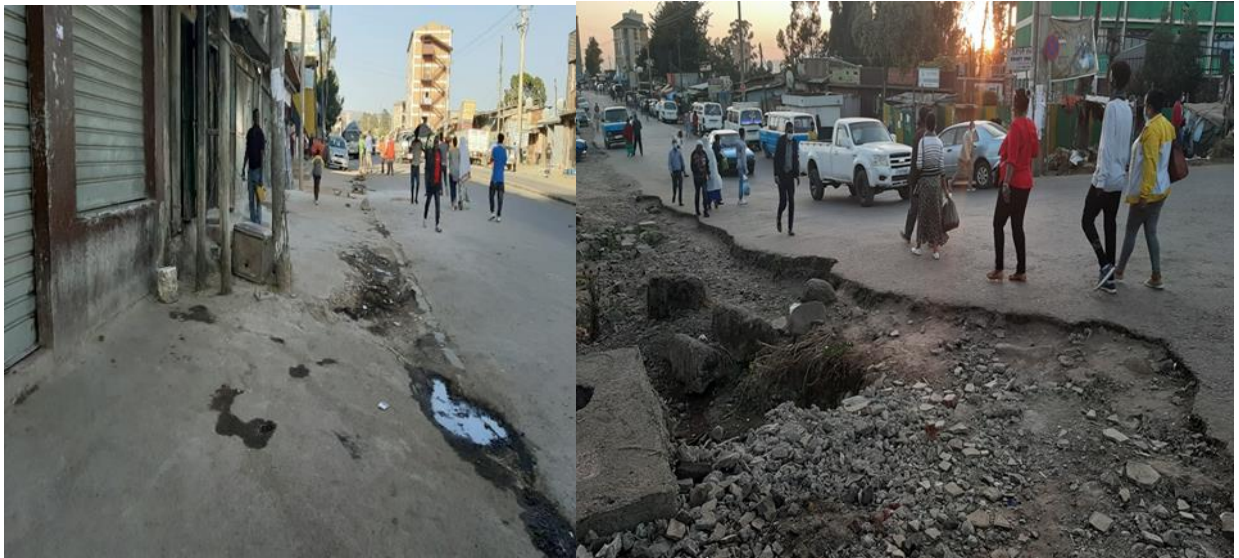
Figure 4. 6: Cracked and damaged pavements
