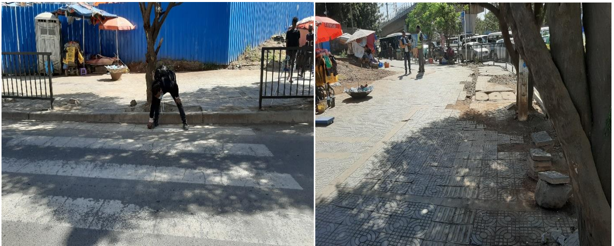
Figure 4. 16: Raised edge at crossing and dismantled tile from walkway
