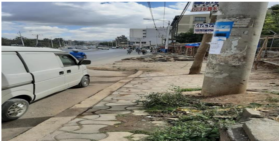
Figure 4. 13: Obstacles on Walkway.
