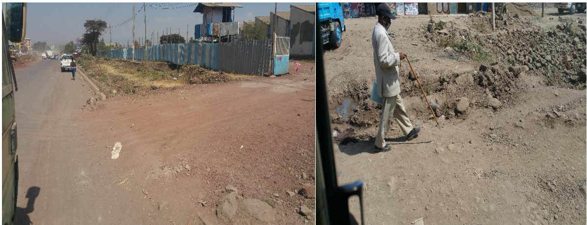
Figure 4. 51:improper walkway and waste materials on road
