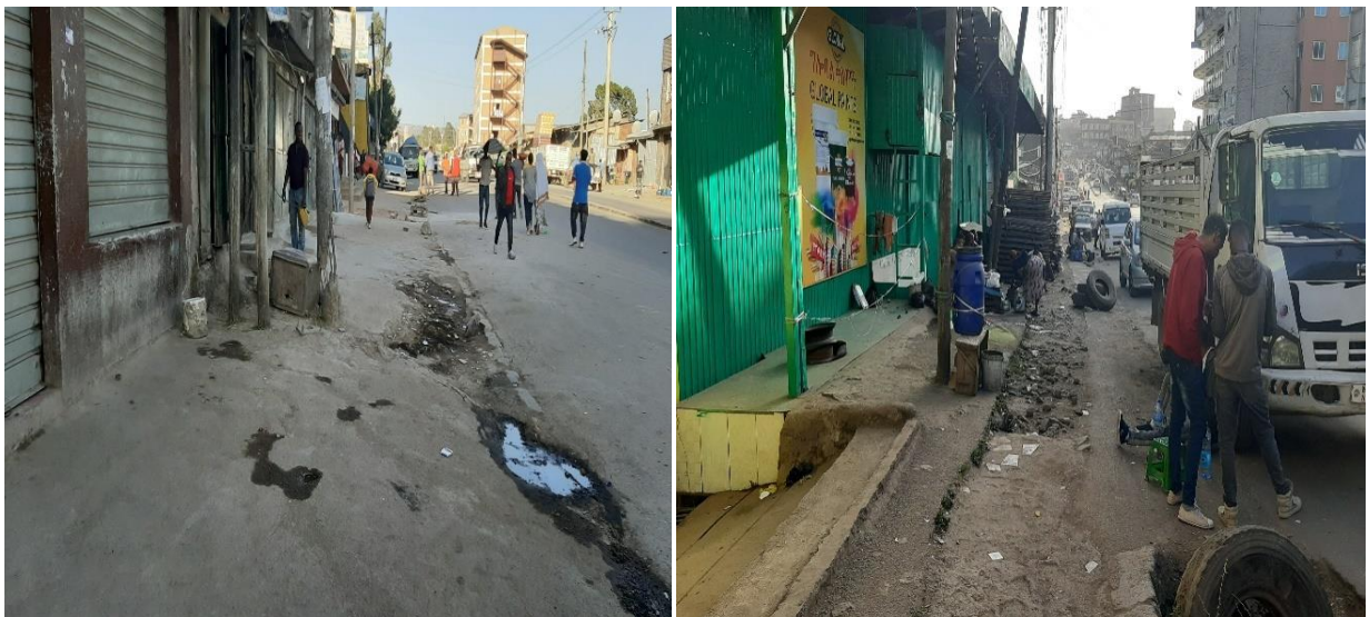
Figure 4. 21: Cracked pavements, unsafe walkways that do not allow passengers to pass and road barriers (telephone poles, liquid and solid waste).
