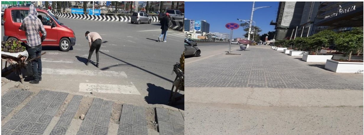
Figure 4. 39:crack of walkway, and trading on pedestrian walk and lack of tactile surface
