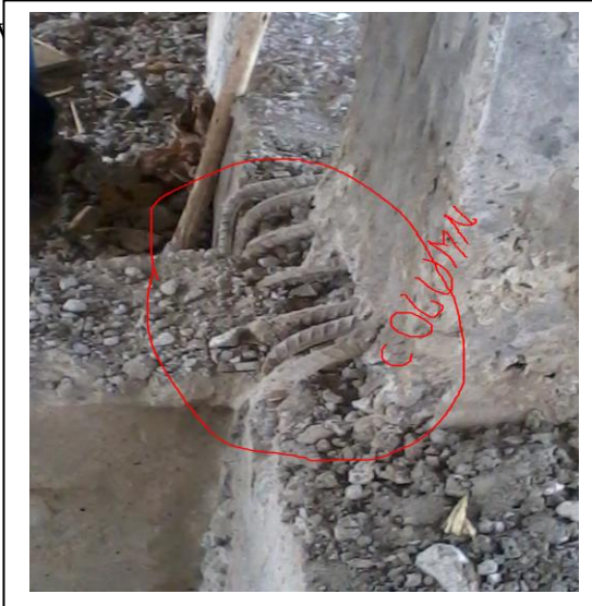
Figure 4.13 Footing columns were not aligned problem to elevation columns
