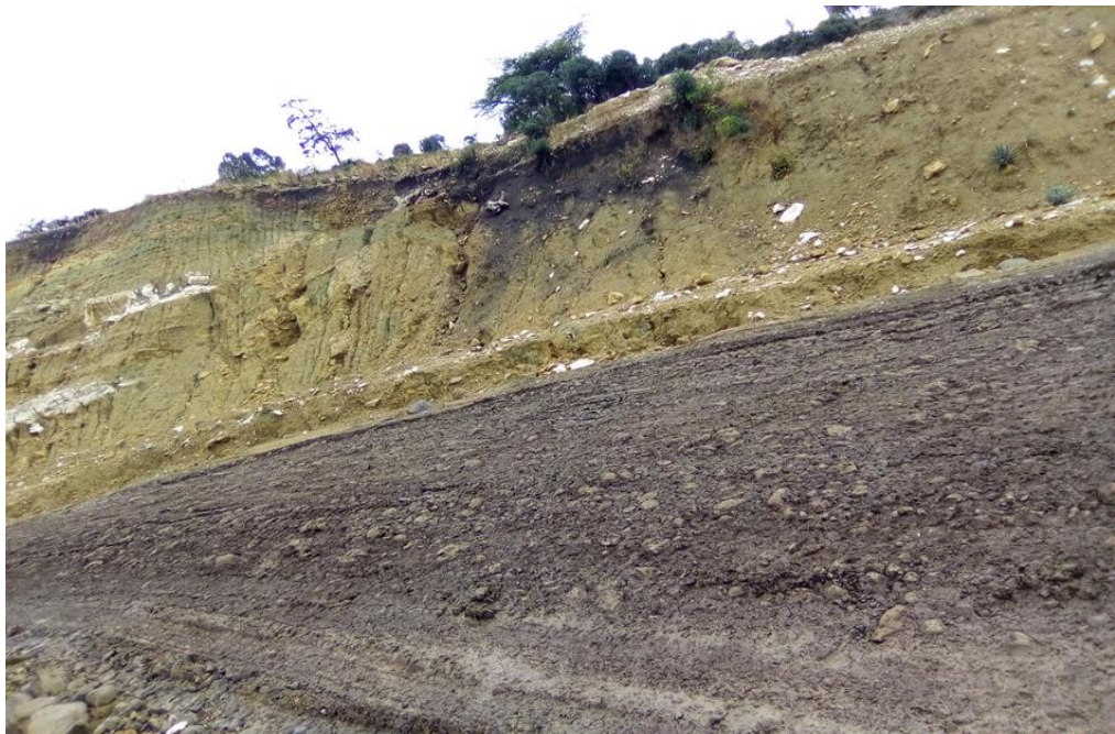
Active land slide photography for existing road
