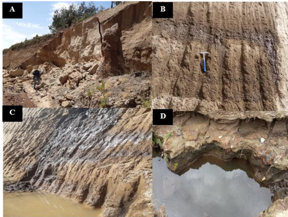
Figure 3. 1 A) Figure showing loose rock falling along the road section, B) evidence of spring on the slope surface, C) Spring called Chefe Hada Ragatu along the road section around Lake Wonchi and D) spring evidence along the road section to Woliso town.
