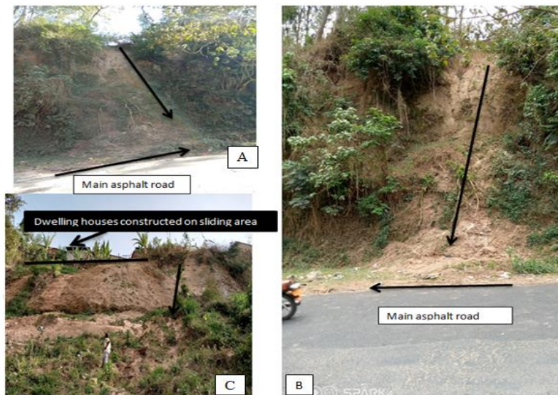
Figure 33: Rotational sliding in the study area on main asphalt road at GPS reading A, (long.433515 m lati. 745683 m). B, (long. 433617 m lati. 745552 m ). C, sliding on dwelling house at GPS reading (long.434401 m lati. 746538 m ).
