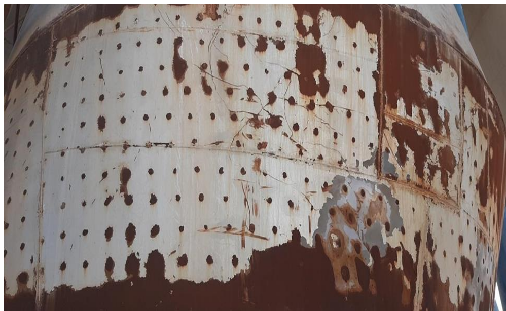
Figure 4.3: Rust area of cyclones exposed to high surface temperature
