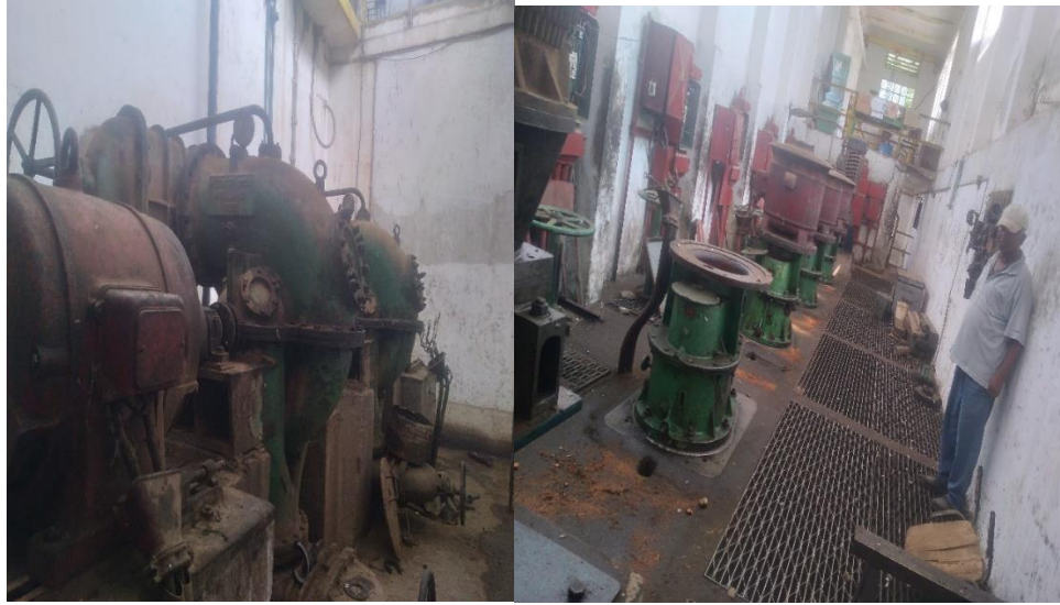
Figure 3.2 Main pump station of Wonji Shoa Sugar Factory
