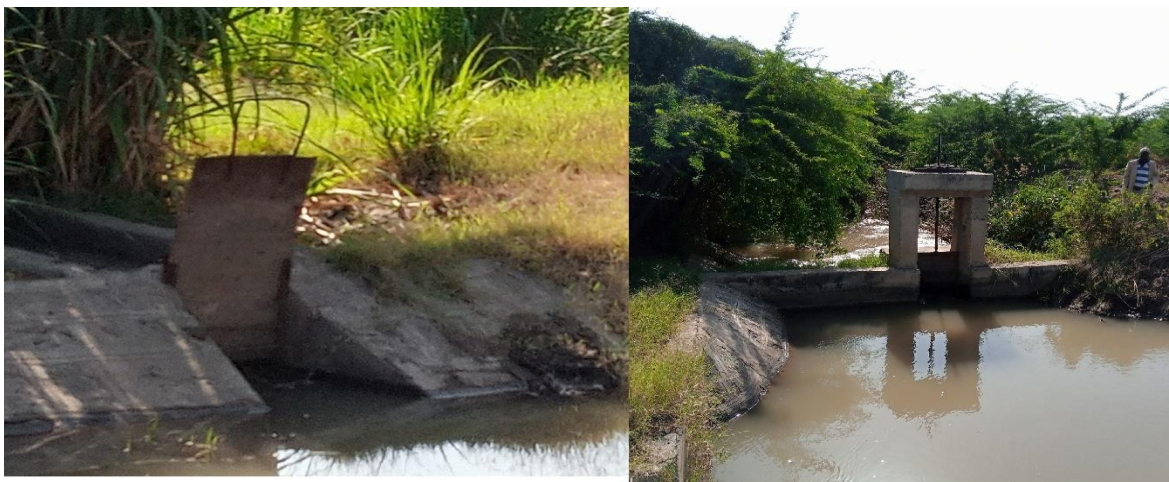
Figure 1.3: Secondary and main canal flow control point
