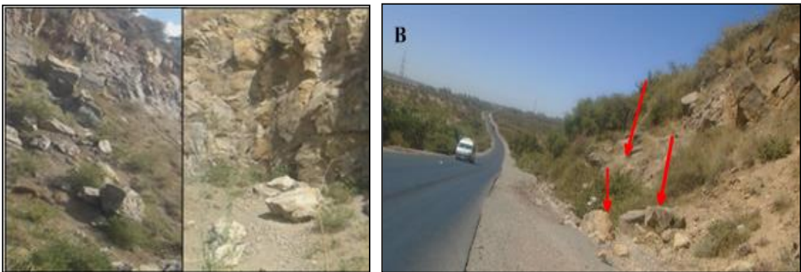
Figure 16: Rock fall in the eastern (left) and south western (right) part of the study area
