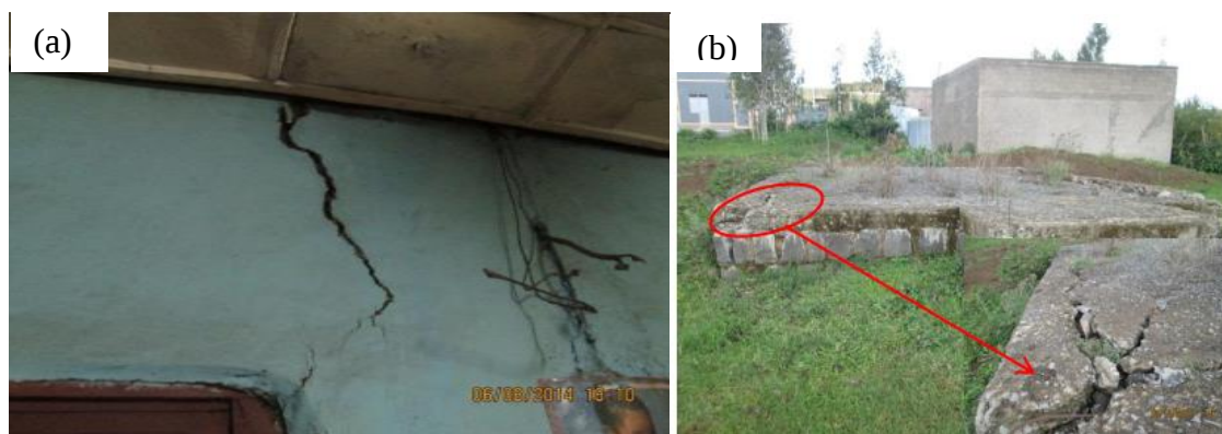
Figure 2.7 Typical damages due to soil swelling and shrinking characteristics show distress on lightweight structures(a,b) (Tibebu, 2015).
