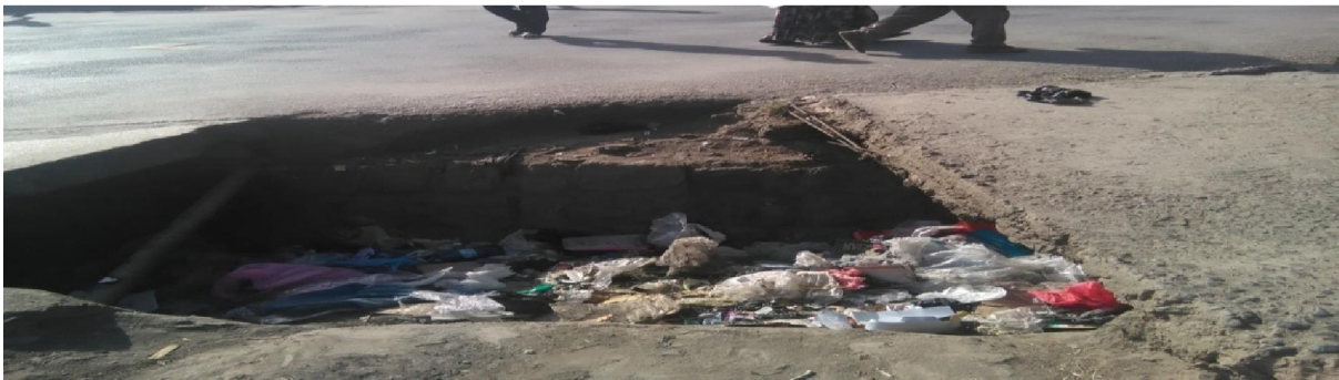
Figure 2.4: Blockage of sewerage systems (photo taken from Adama city around bus station)
