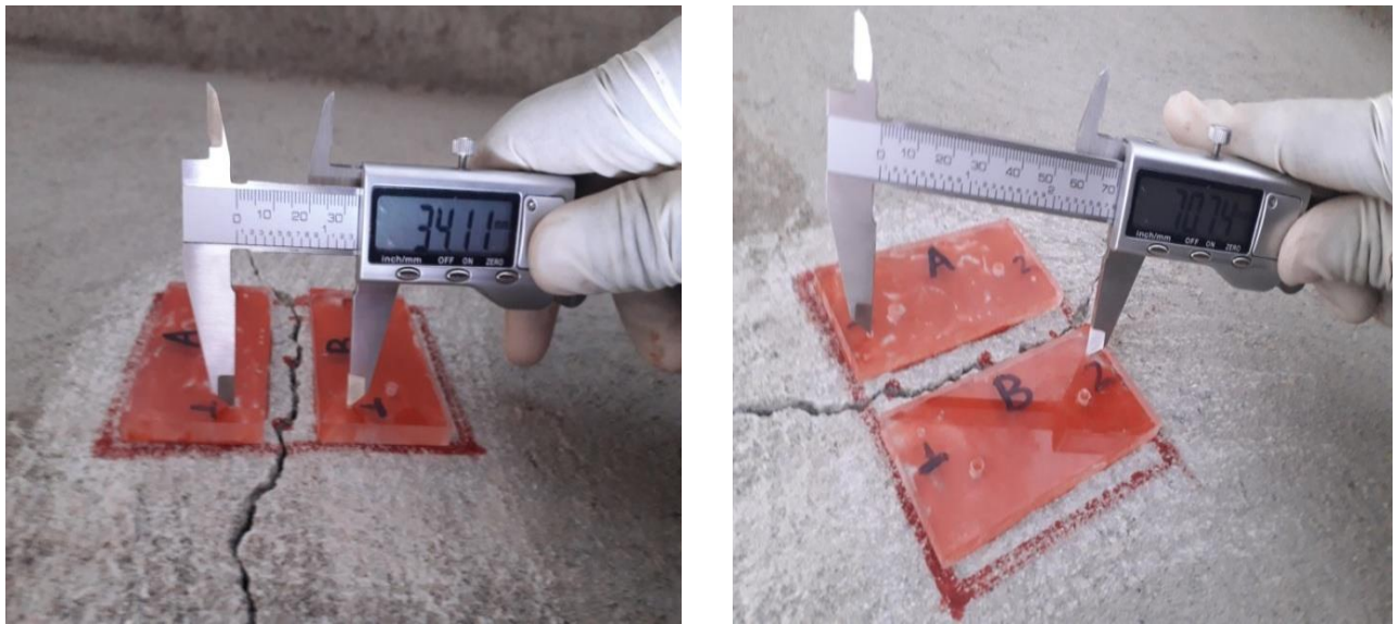
Figure 4. 13: 2D crack monitor measuring across and along the crack Building ID No.26
