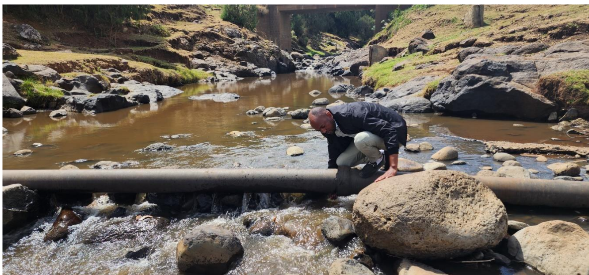
Figure 4. 10: Amereba Indato Pipe laying without any support of pipe line
