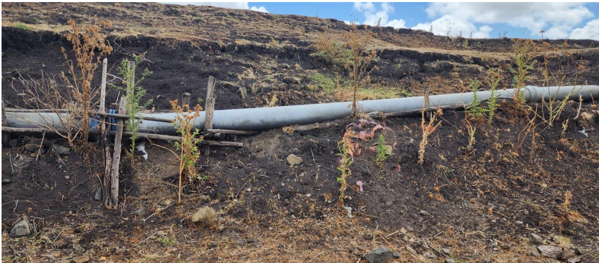
Figure 4. 11: Amereba Indato water supply of pipe line affected by Soil erosion
