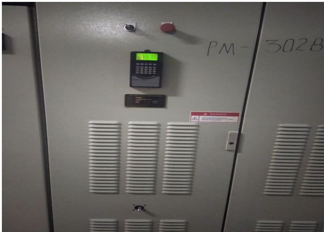
Figure D.3 VFD controller installed with control panel of the kiln motor drive
