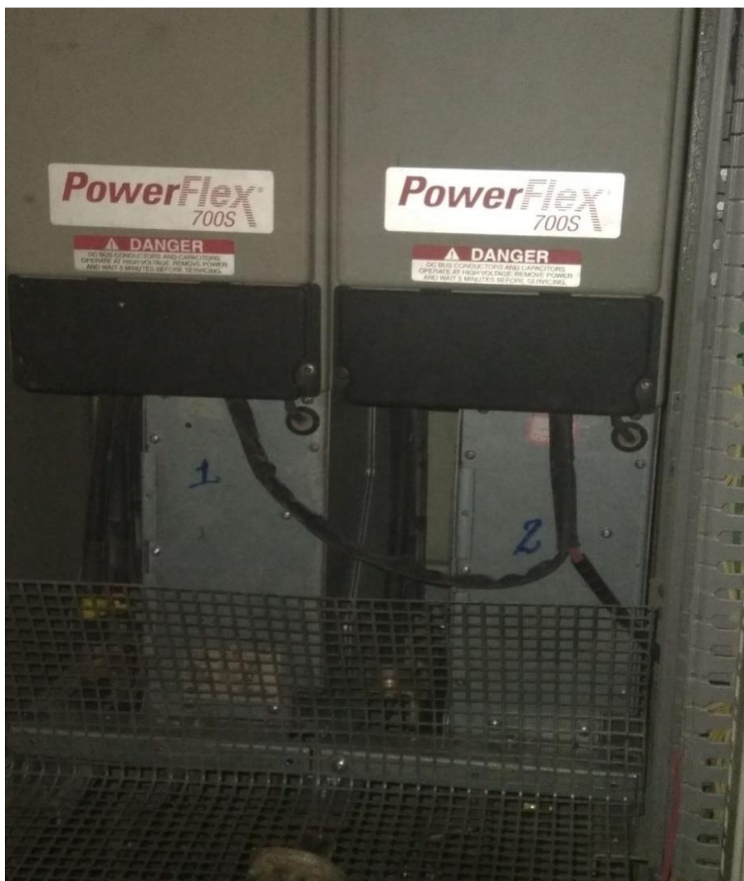
Figure D.4 Adjustable Frequency AC Drive for kiln motor drive system
