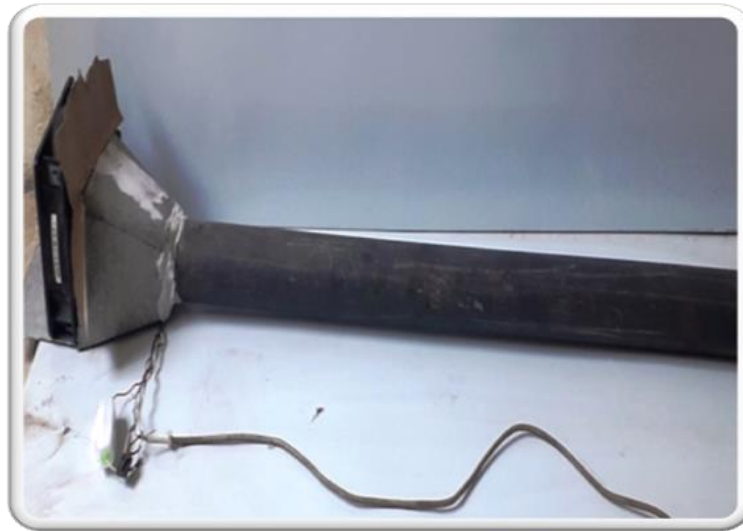
Figure 3.7: Air Supply System
