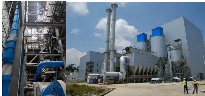
Figure 4: Reppi Waste to Energy facility boilers and Waste to Energy Plant of Reppi
