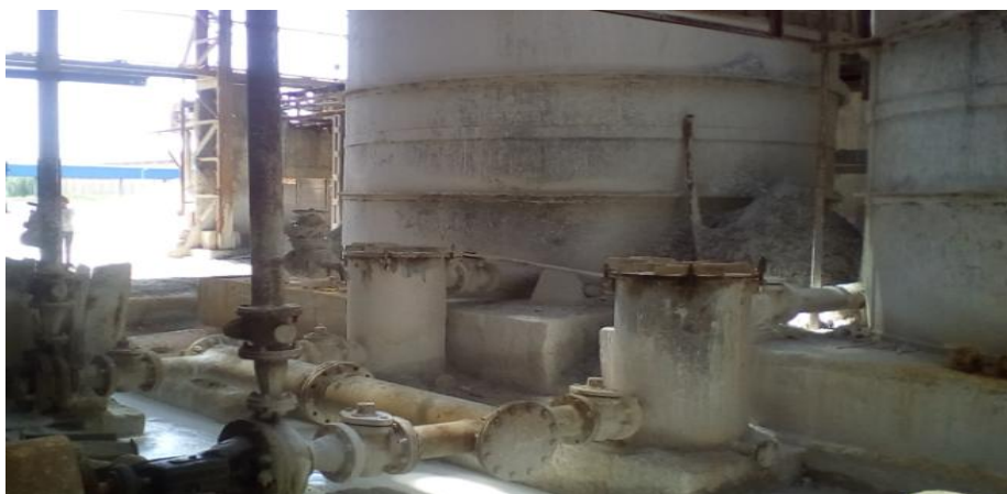
Figure 5: Milk of Lime storage and pumping station (Wonji Shoa Sugar Factory)
