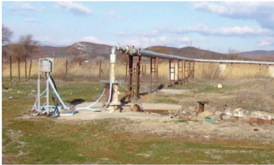
Figure 36: Aboveground geothermal pipeline in Smokvica, Macedonia (Sanja et al., 2011)
