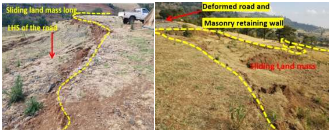
Figure 3.10 side slopes failures at Site-11(Reference Author)
