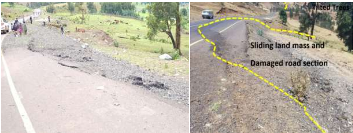
Figure 3.4: The typical rotational embankment failure at Site-3(Reference Author)
