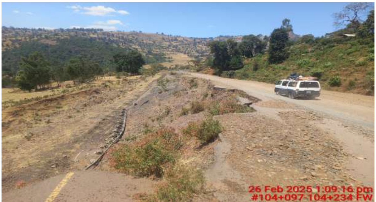
Figure 3.8: The typical rotational embankment failed at Site-7(Reference Author)
