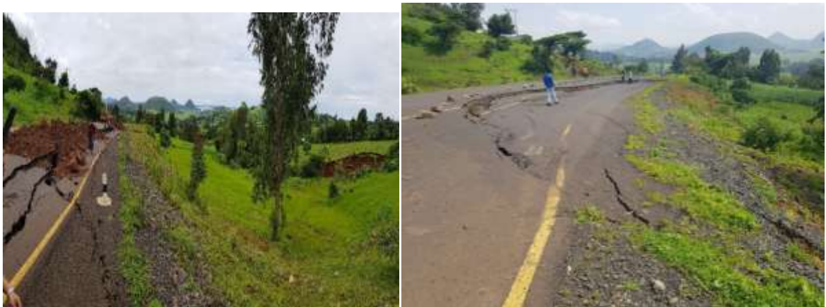
Figure 3.3: The typical rotational embankment failure at Site-1(Reference Author)
