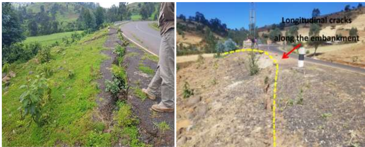
Figure 3.5: The typical rotational embankment failure at Site-5(Reference Author)
