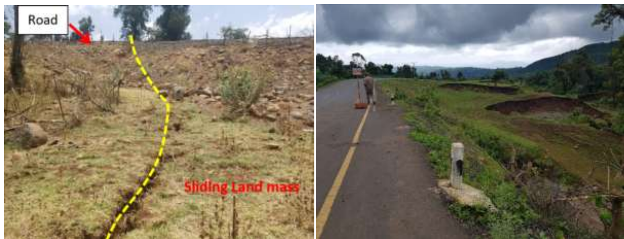
Figure 3.9: The pavement and embankment failures in Site-9(Reference Author)
