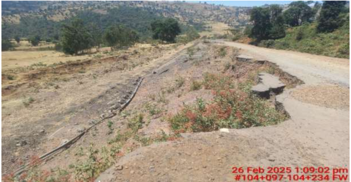
Figure 3.7: The typical rotational embankment failed at Site-7(Reference Author)
