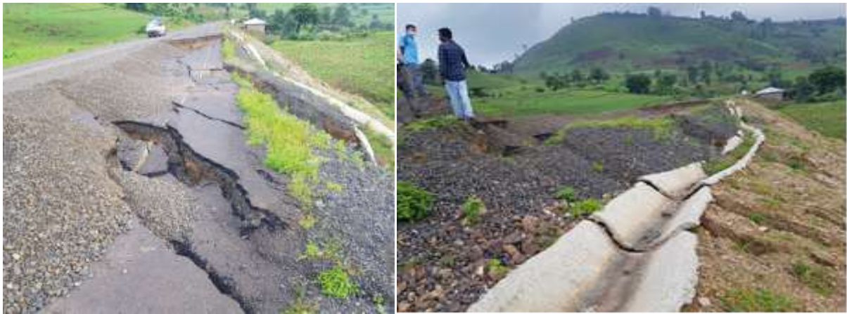
Figure 3.6: The typical rotational embankment failure at Site-6(Reference Author)
