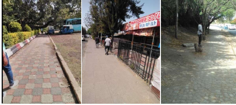
Figure 4.13: Site pictures of the sidewalk conditions; Source: (Own Researcher, 2022)
