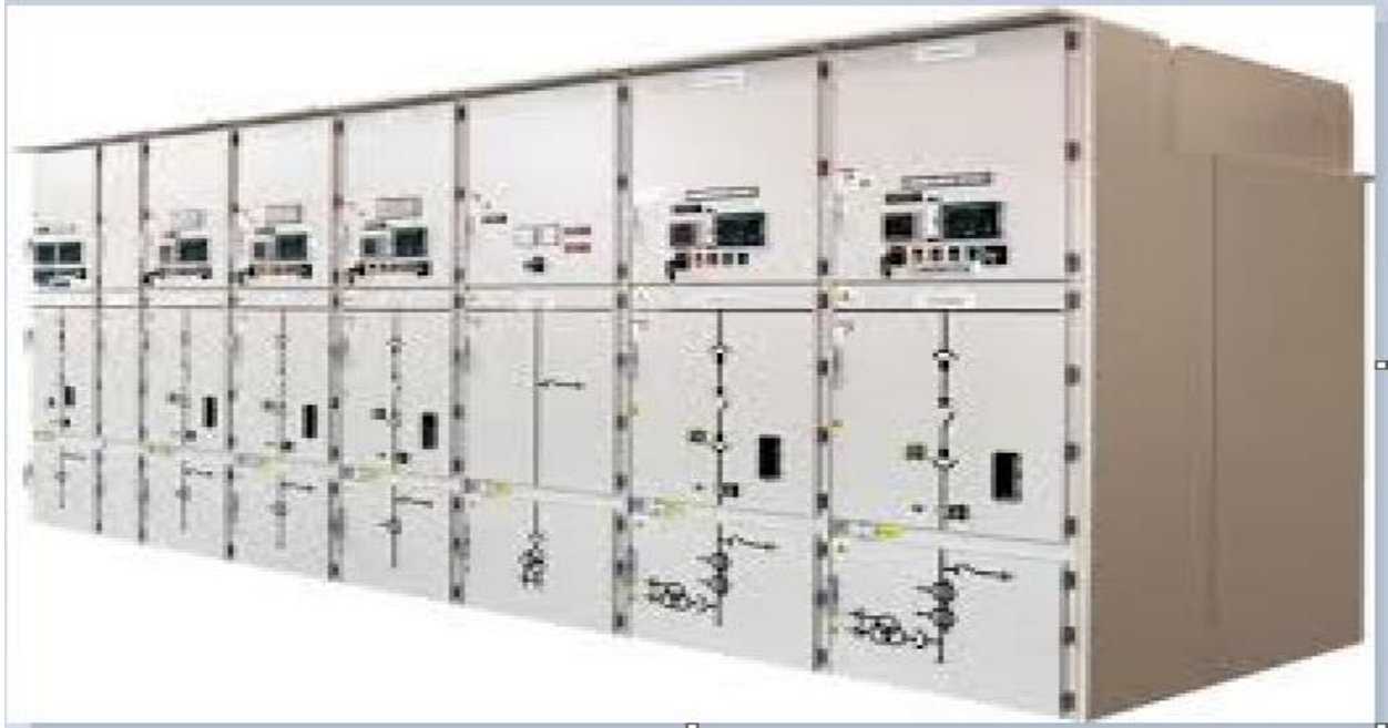
Figure 4.5. Power plant switchgear 11kv bus bar
