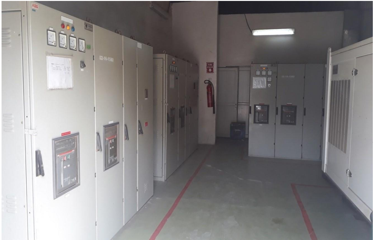
Figure.1.4.Distribution system CMDB boards for Adama Spinning Factory
