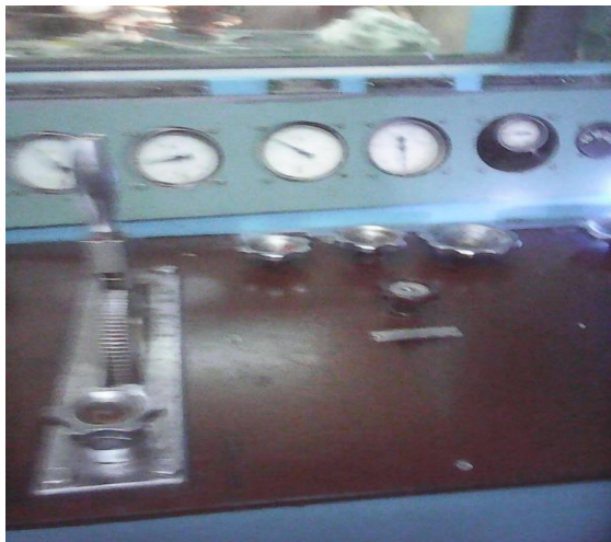
Figure A3: Temperature and pressure gauge
