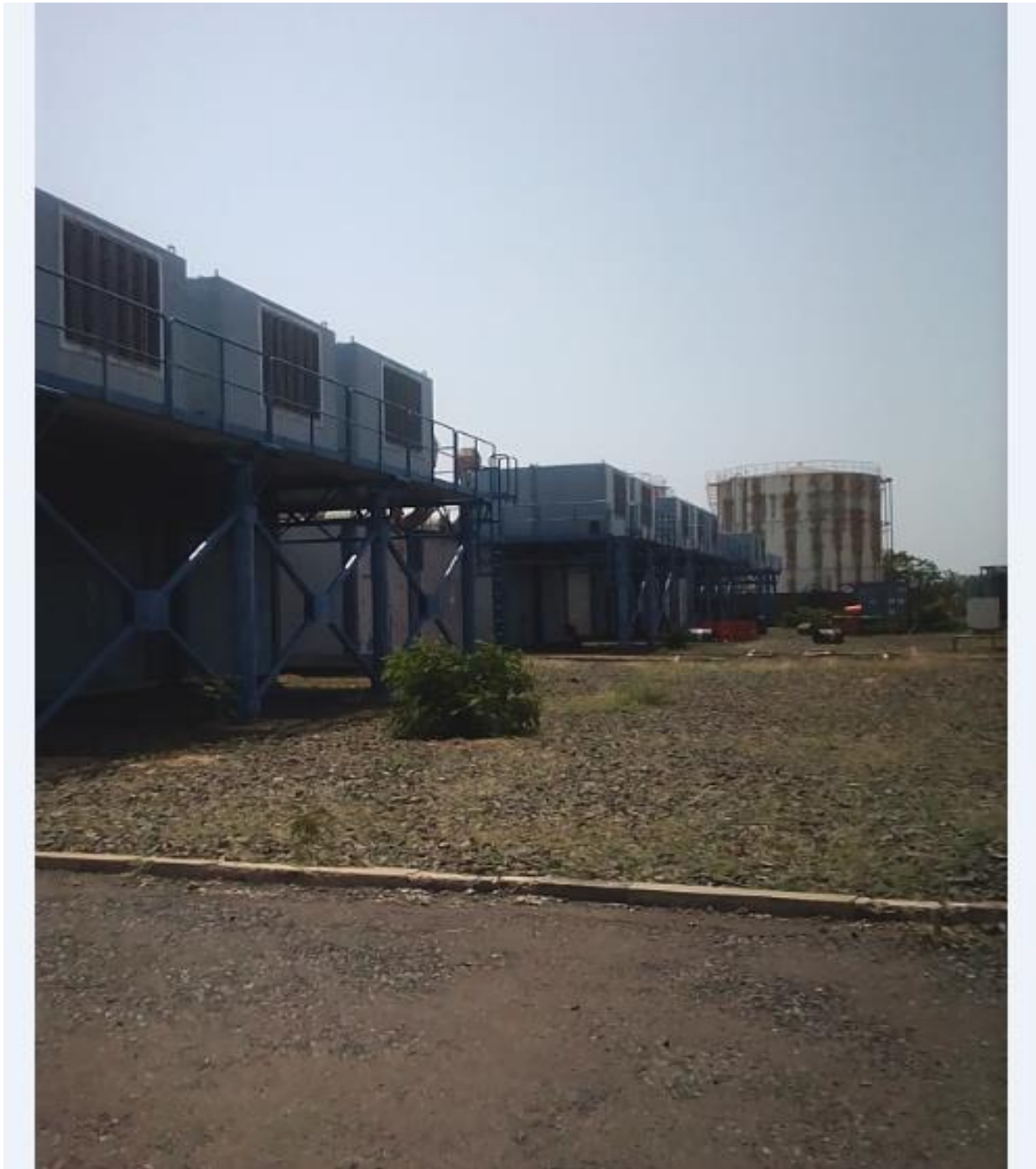
Figure 3.4: Awash7 Diesel Substation
