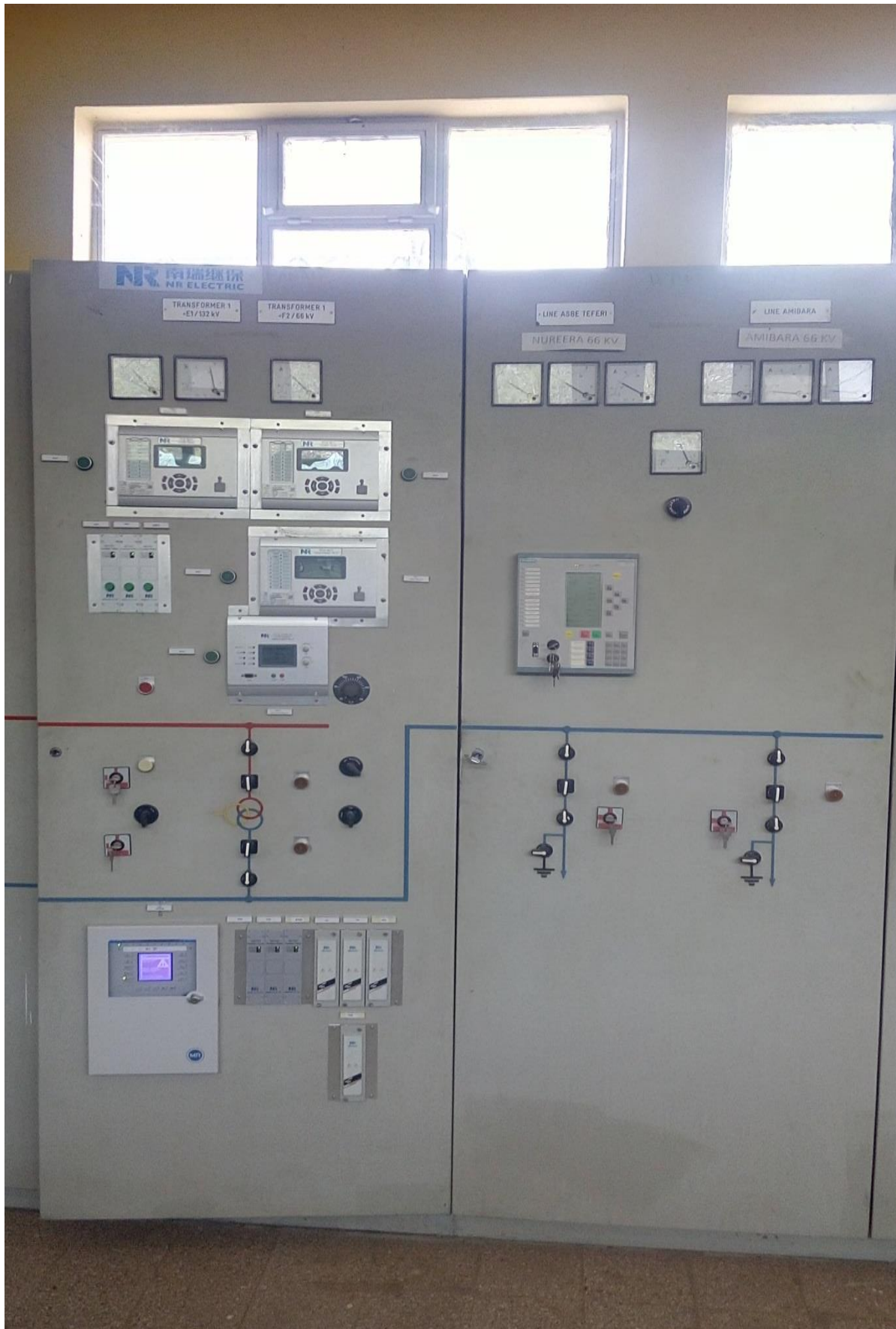
Figure 3.2: Partial view of Awash7 kilo Substation Control Room [Source: study area]
