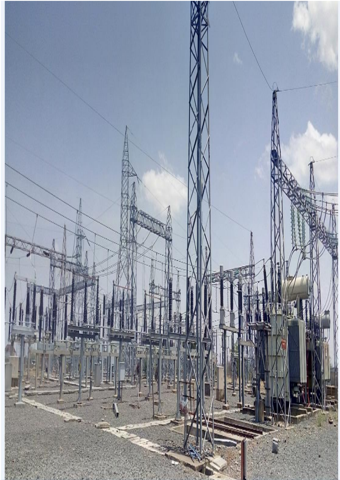
Figure 3.3: Awash7 kilo Substation [Source: study area]
