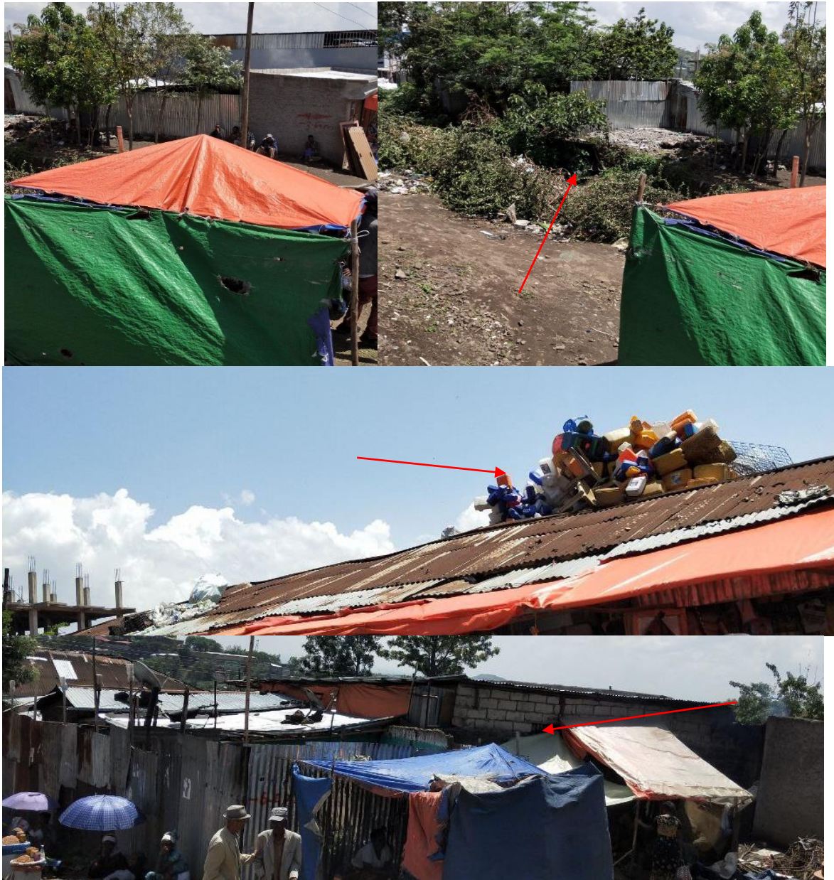
Figure: 4.19. Bad housing condition in different site of study area.
