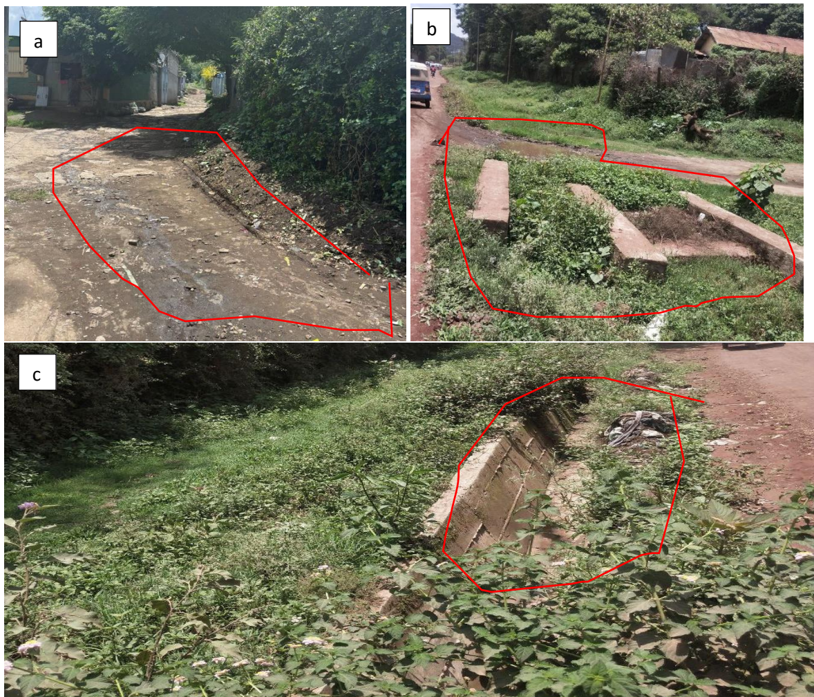
Figure 4.12 (a) village lack of drainage without /no drainage line used road as drainage. (b) drainage line blighted area (c) Partially Ditches filled with silt and solid wastes and rain water collected. (Source: photo by the author, 2024)
