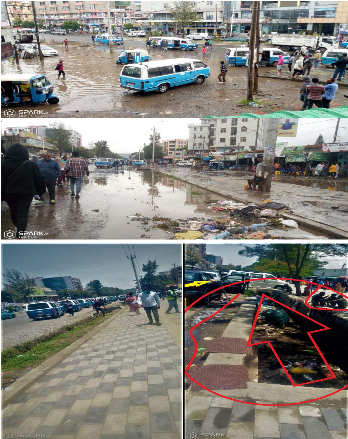
Figure C.4. Photo no zebra crossing, no properly constructed side walkway, no guard fencing or safety barrier on the ditch at Warka.
