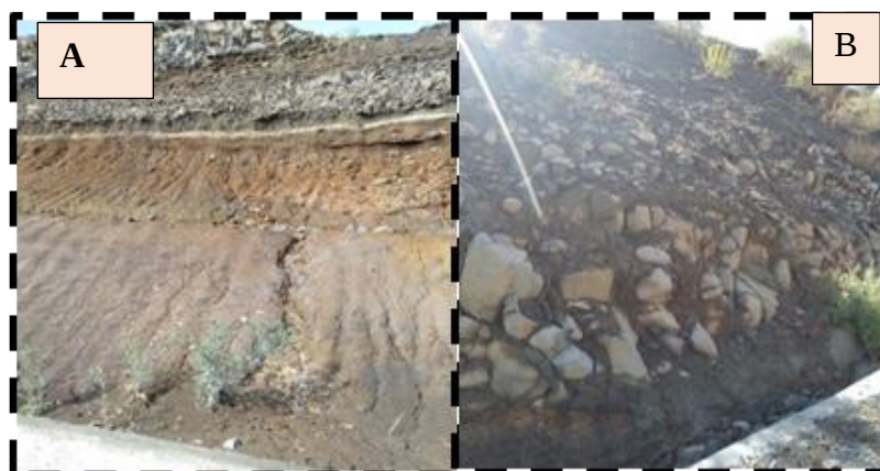
Figure 3. 2: Critical slope sections a) Heterogenous critical slope (welded scoria-colluvial material-aphanitic basalts) R1SS and b) Heterogenous critical slope two (aphanitic basalts-vascular basalts- scoria) R2SS1 which are filled by soil due to erosion problems
