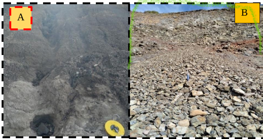
Figure 3. 6: A) Slope section of soil sample (SS3) and B) Circular failure of highly weathered basalts from bench two
