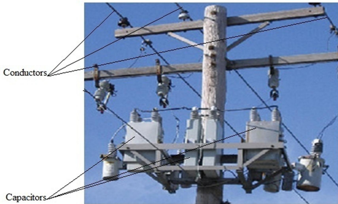
Figure 2.6 Pole mounted medium voltage capacitor
