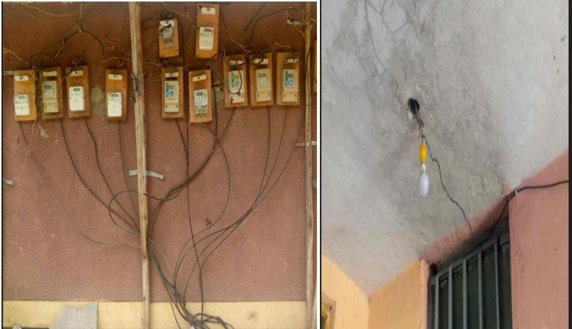
Figure 4. 5: Adequate electrical system maintenance
