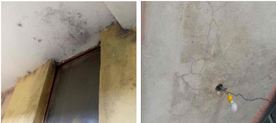
Figure 4. 13: Dampness and Moisture
