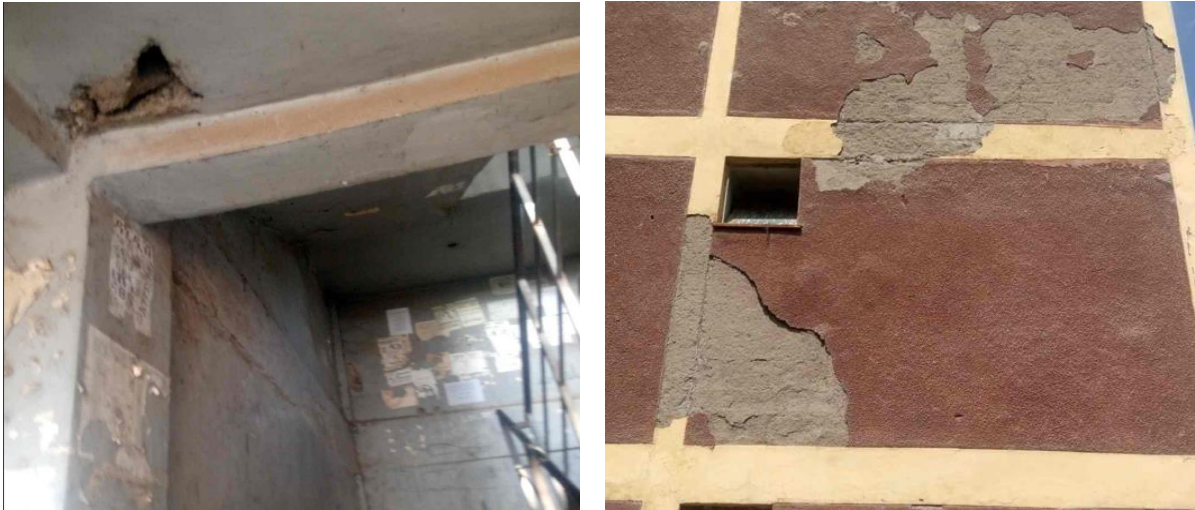
Figure 4. 12: Poor Construction Workmanship
