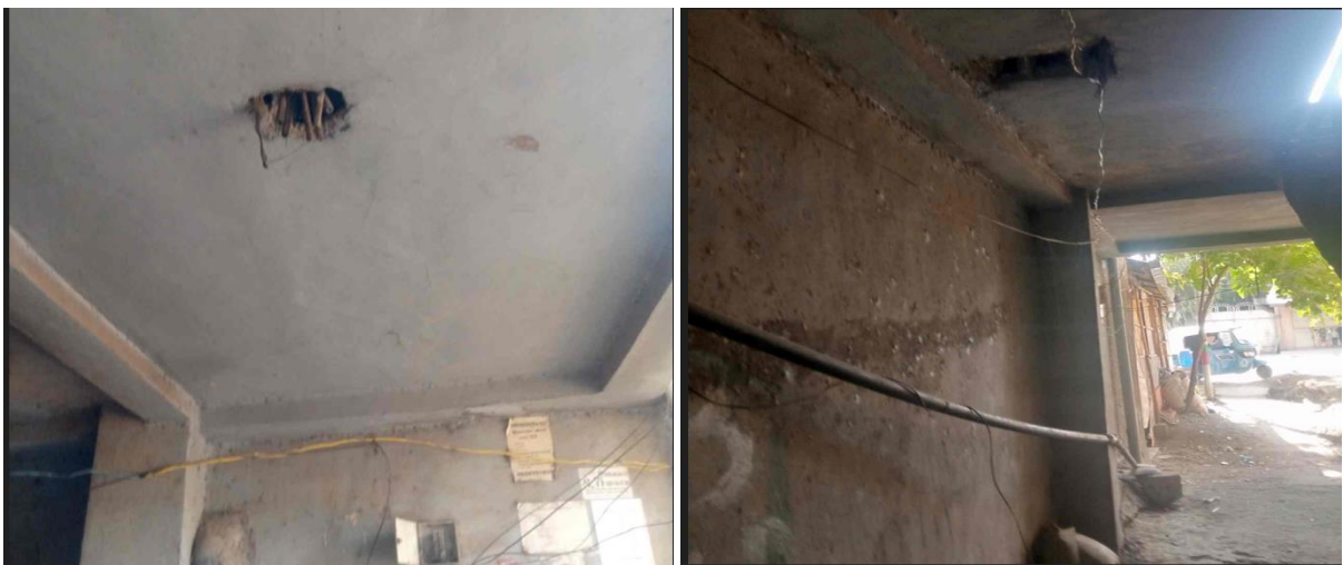
Figure 4. 9: Electrical Work Problems
