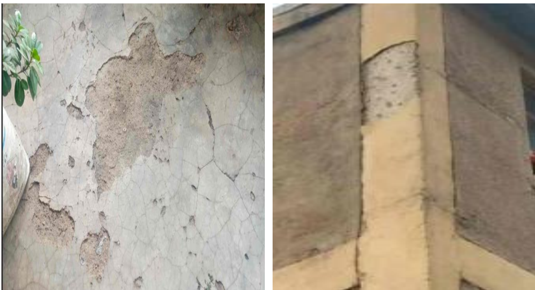
Figure 4. 3: Quality of construction workmanship
