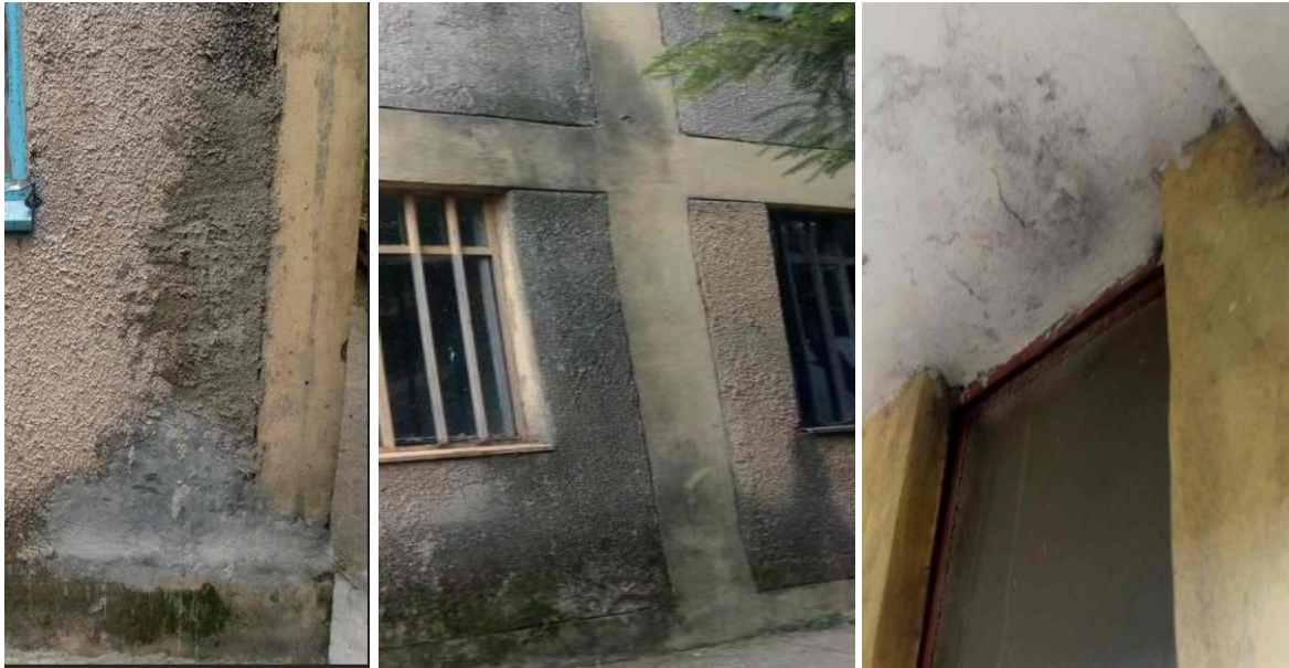
Figure 4. 2: Moisture and mold
