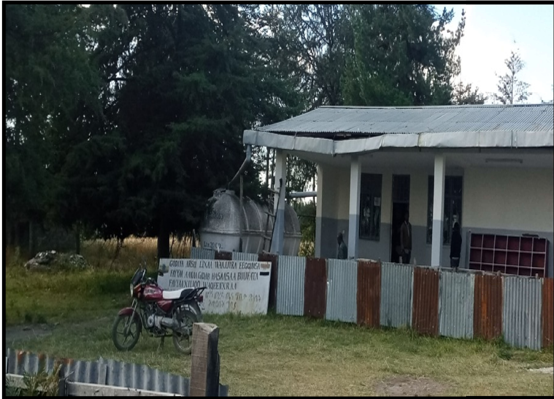
Figure 12: Gutter dismantled and dumped out at Observation point 2; September, 2022
