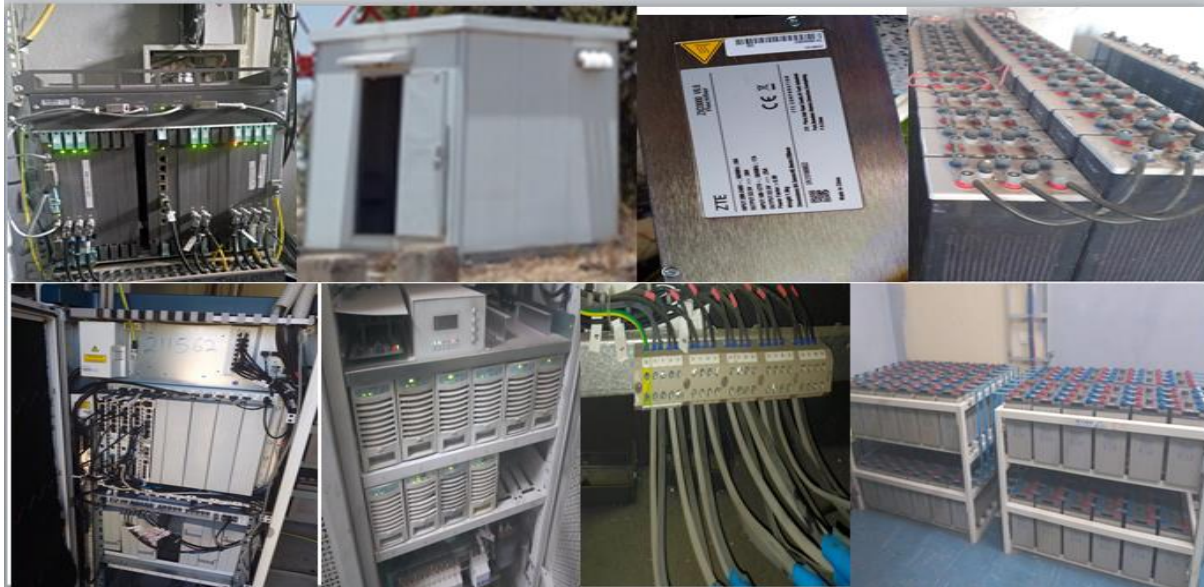
Figure 3.1 Existing Indoor Equipment pictures taken from Site 211367 & 211562, March 2022
