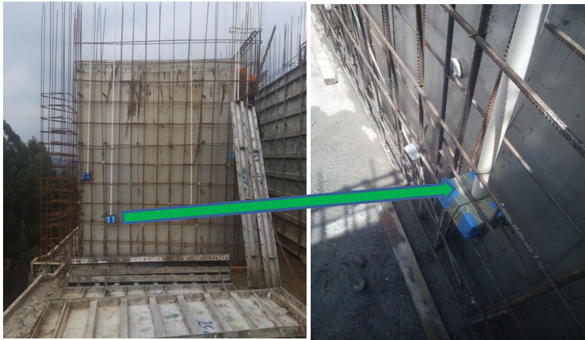
Figure 4. 8: Electrical installation inside wall Switch and socket points
