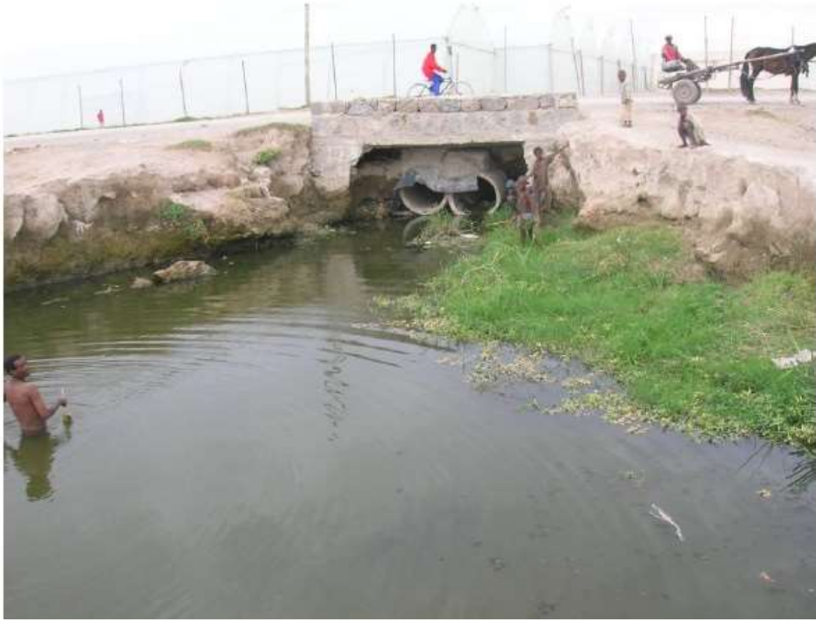
Photo 11: Drainage disposal at share Ethiopia to the Lake Zeway
