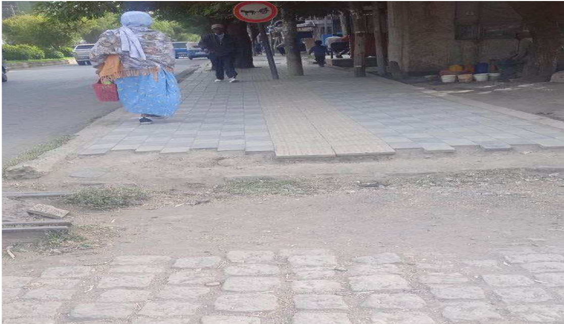
Figure 4.4. Walkways lacking continuity and access ramps
