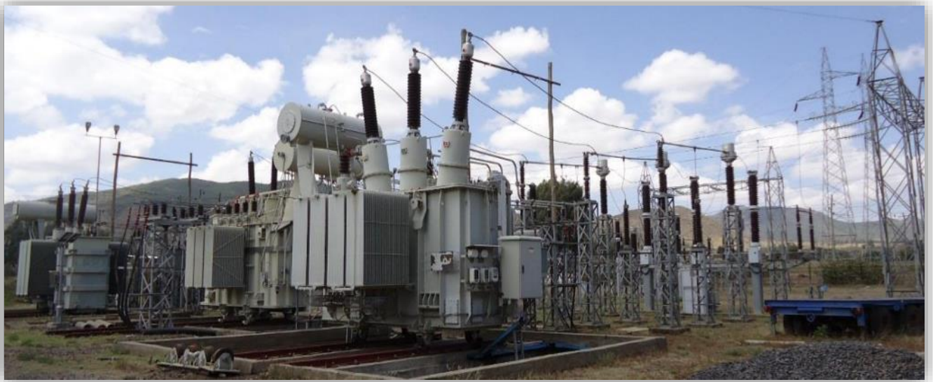
Figure 1.2: Bishoftu substation II taken during site visit
