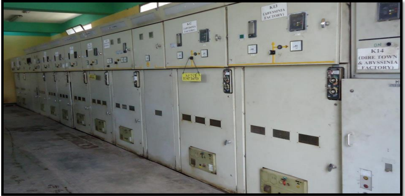
Figure 1.3: Control room of Bishoftu substation II
