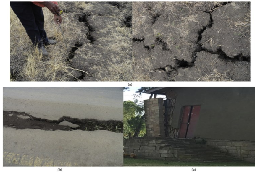
Figure 1: (a) Typical cracks in BC soil during the dry season, (b) Typical crack scene on roads around Ambo, and (c) Serious damage on a house constructed on BC soil (M.K. Atahu, 2018)
