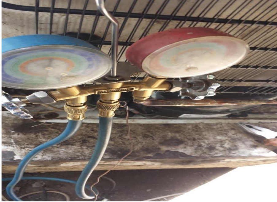
Figure 4.5: Measuring the pressure of the refrigerator
