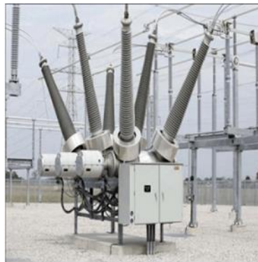
Figure 4.14: Circuit breaker in substation [33]
