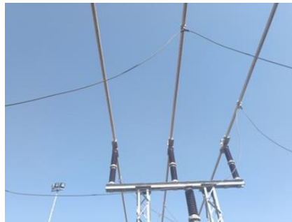
Figure 4.12: Bus bar in substation [33]
