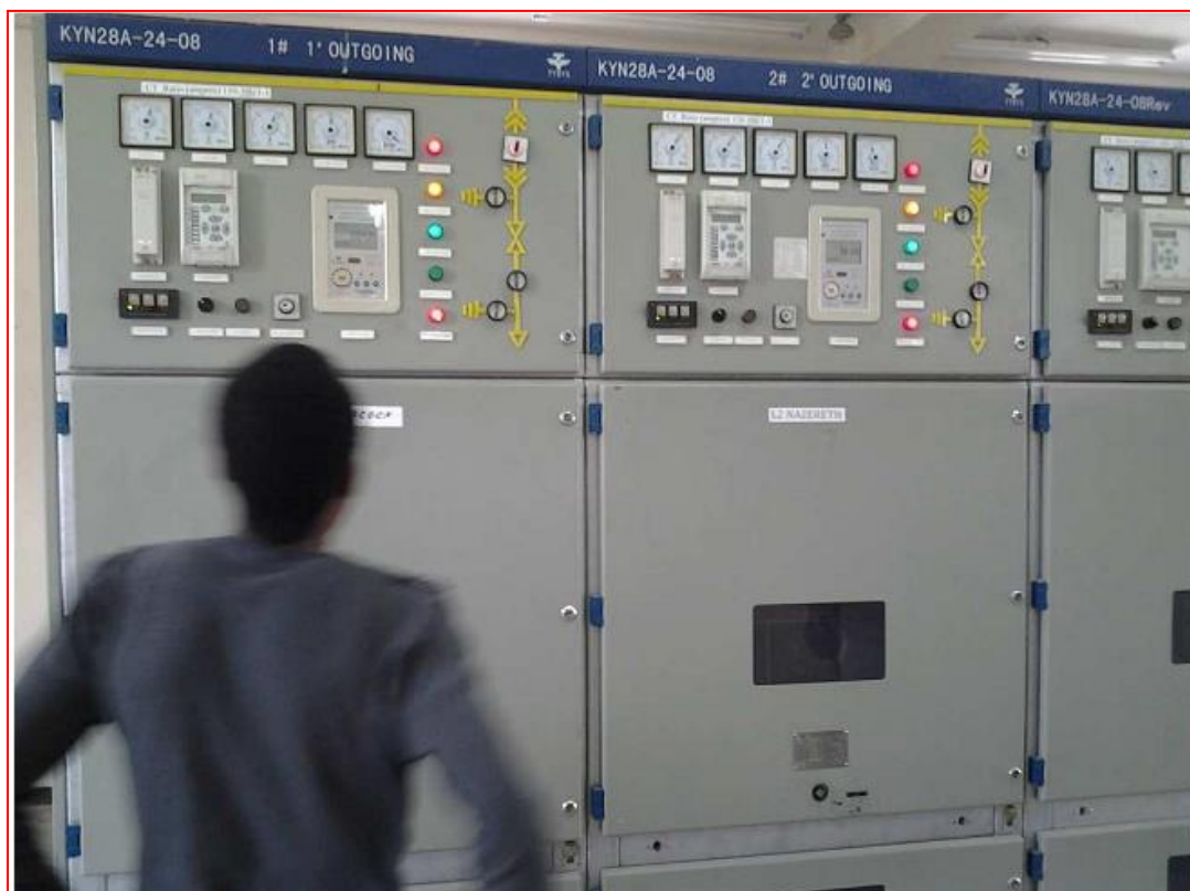
Figure 4.5: Adama Substation 15kV switchboards with 630A
