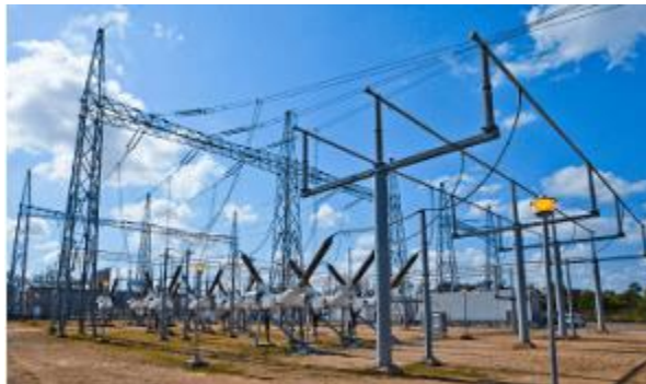
Figure 4.16: Switchyard in substation [33]
