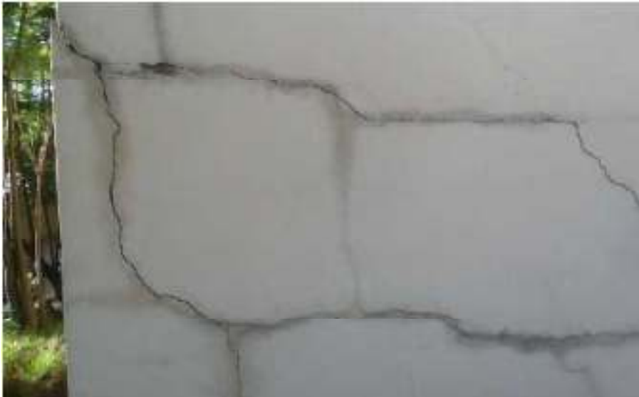
Figure 1. Wall crack on Block 2, Right wing
