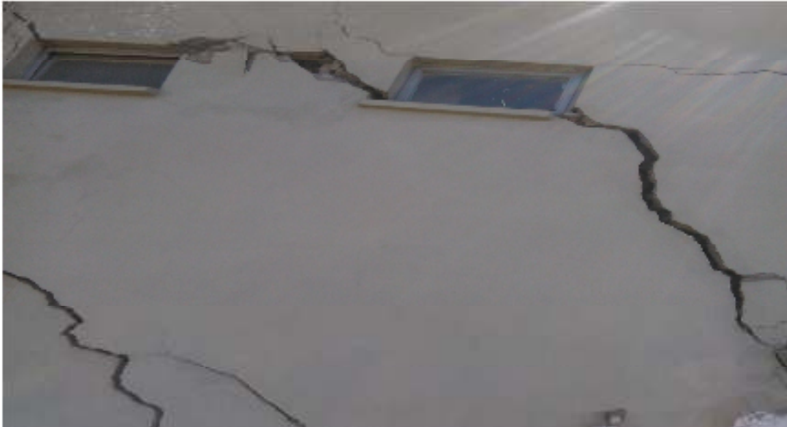
Figure11.Serious wall crack around window on multi –purpose hall
