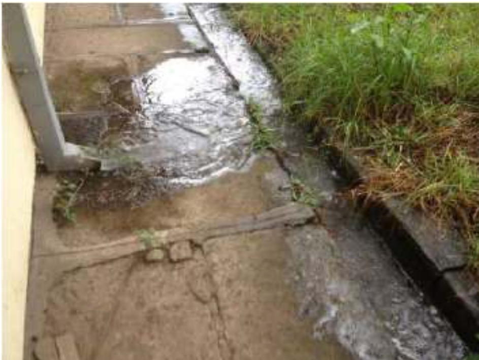
Figure3. Percolation of rainwater from down pipe through separation of Walkway and non-functional side ditch to underneath of the building on
