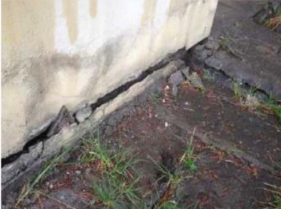
Figure 2. Separation of super structure with the peripheral masonry and Walkway on Block 2, left wing
