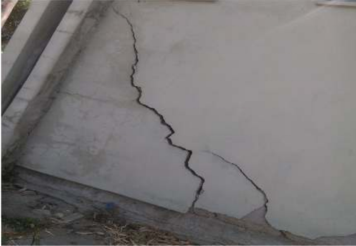
Figure 13. Serious wall crack and separation of beam to foundation masonry on multi –purpose hall
