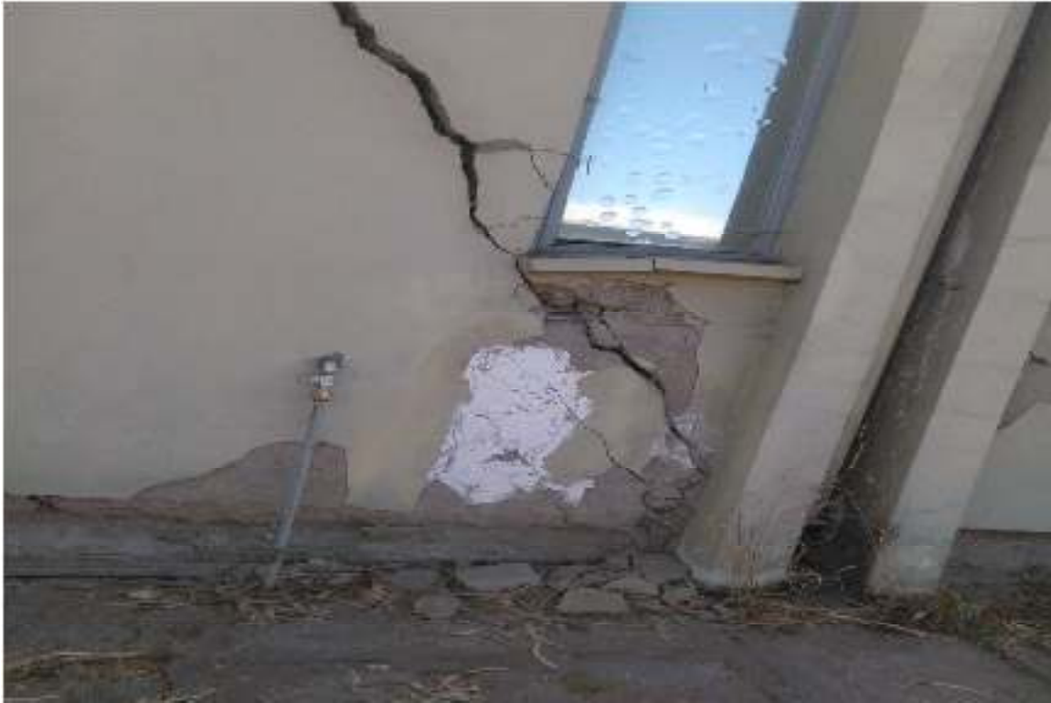
Figure 12. Serious wall crack and separation of beam to foundation masonry on multi –purpose hall
