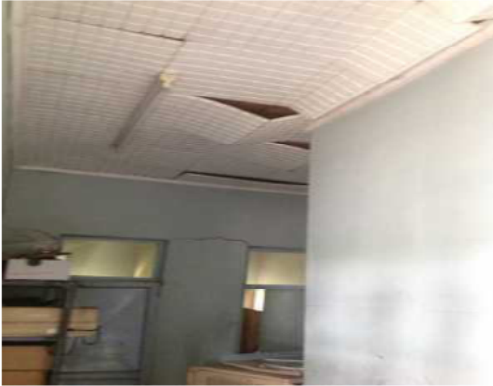
Figure 8. Bending of Ceiling Block -4
